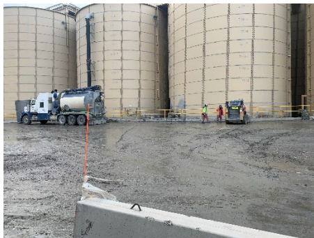
Figure 5. Spill clean up photograph (Jan 31)
