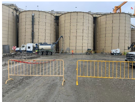
Figure 6. Spill clean up photograph (Jan 31)
