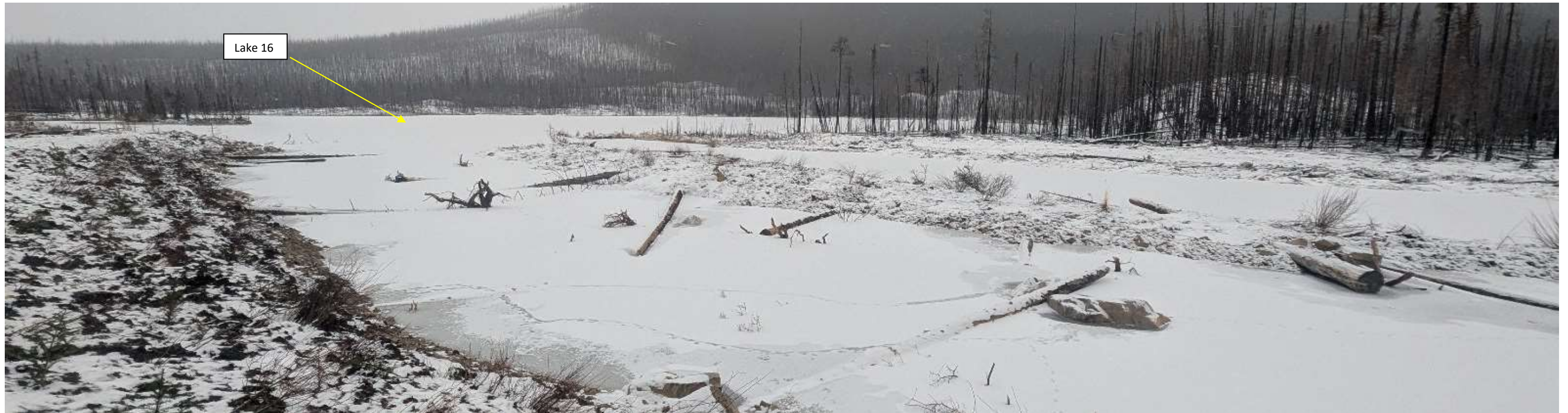
Photo 114724-2. Overview of recent works completed on the Lake 15/16 fish habitat offset channel (near the lake 16 outlet). Works included channel widening, placement of woody debris and rock for habitat complexity, and seeding and willow staking of shoreline in foreground of photo.
