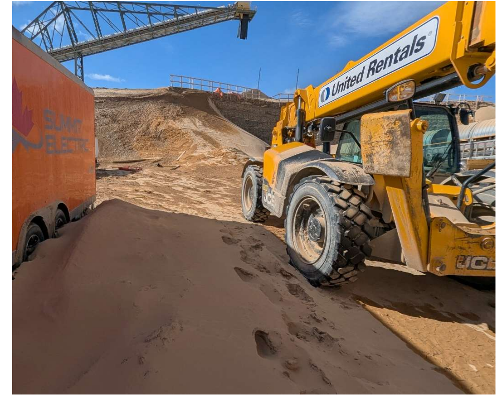
Photo 113338-5. Example of high-grade ore dust accumulation on top of snow at the Plant Site on March 18, 2025.
