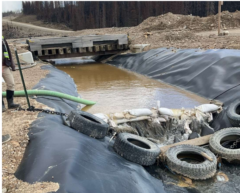
Photo 113688-1. Water flow within the south collection ditch which passively discharges into the CWTP. When turbidity levels become elevated, water can be pumped directly to the tailing's storage facility (via the pump line in place in photo).
