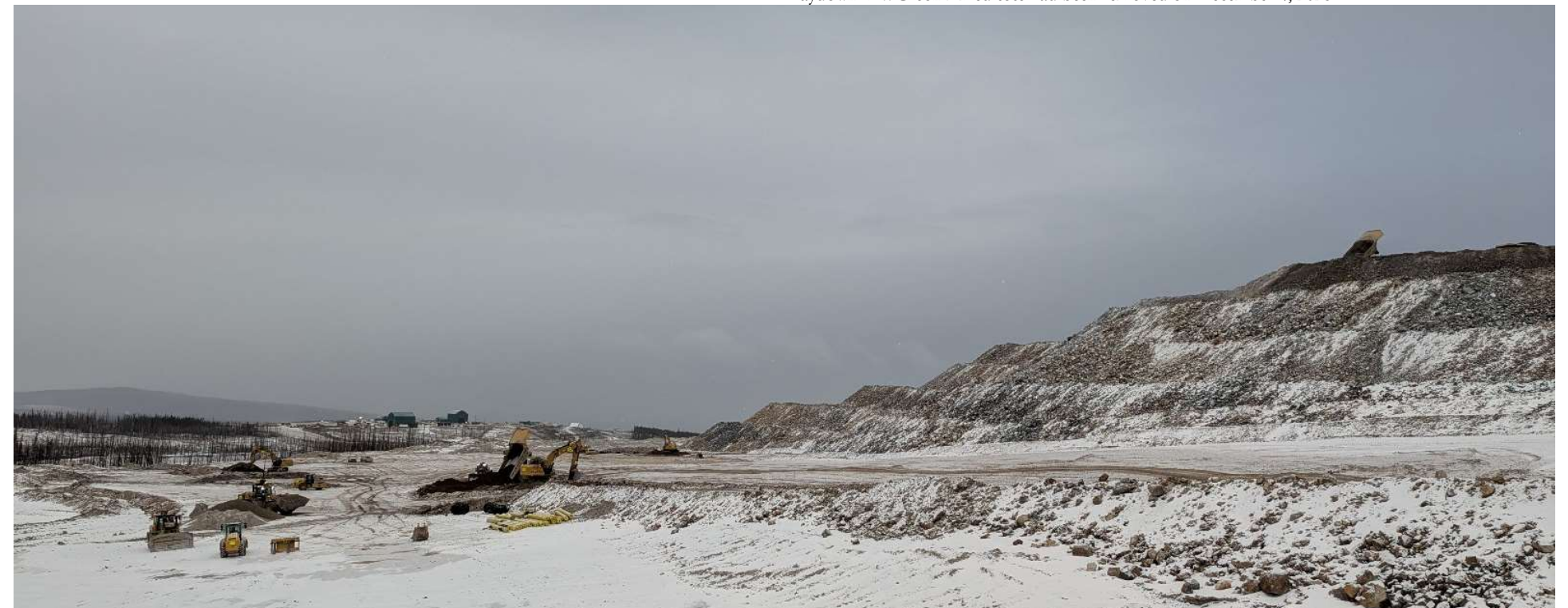
Photo 114716-2. Overview of development of the western end of the low-grade ore stockpile pad (installing compacted base and drainage channels). Low grade ore placement continues at the existing stockpile within the footprint of the previously constructed portion of the pad (with compacted base and water management features).
