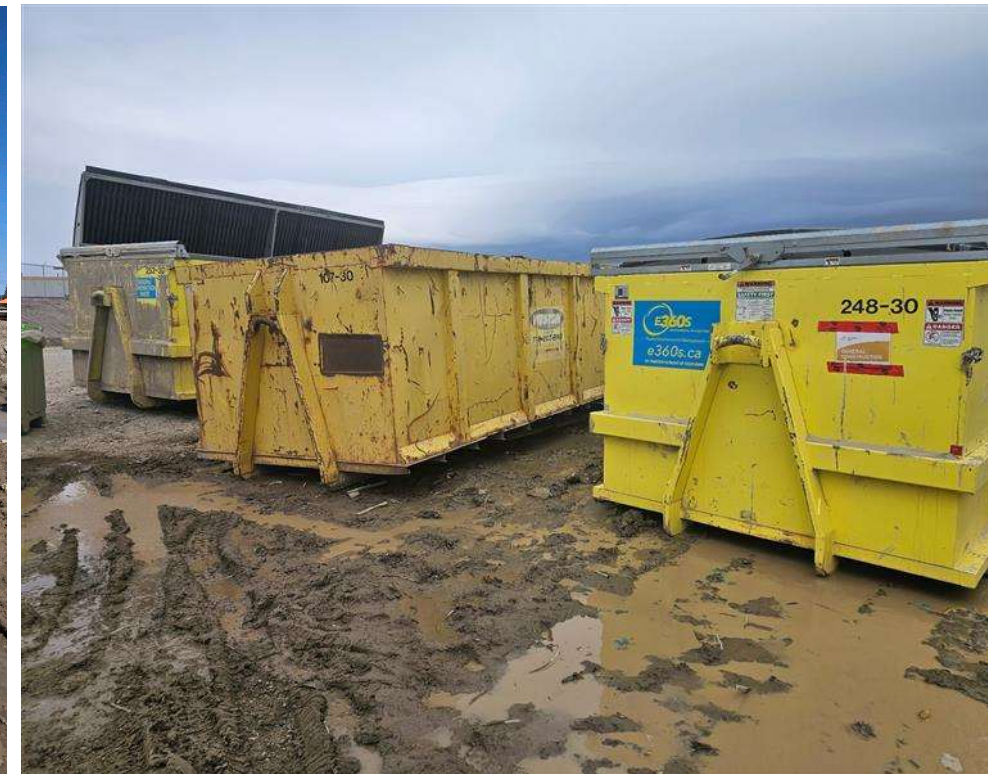
Photo 5. Construction waste bins at the Plant Site following clean up by BWG. Photograph provided by BWG on April 23, 2025.
