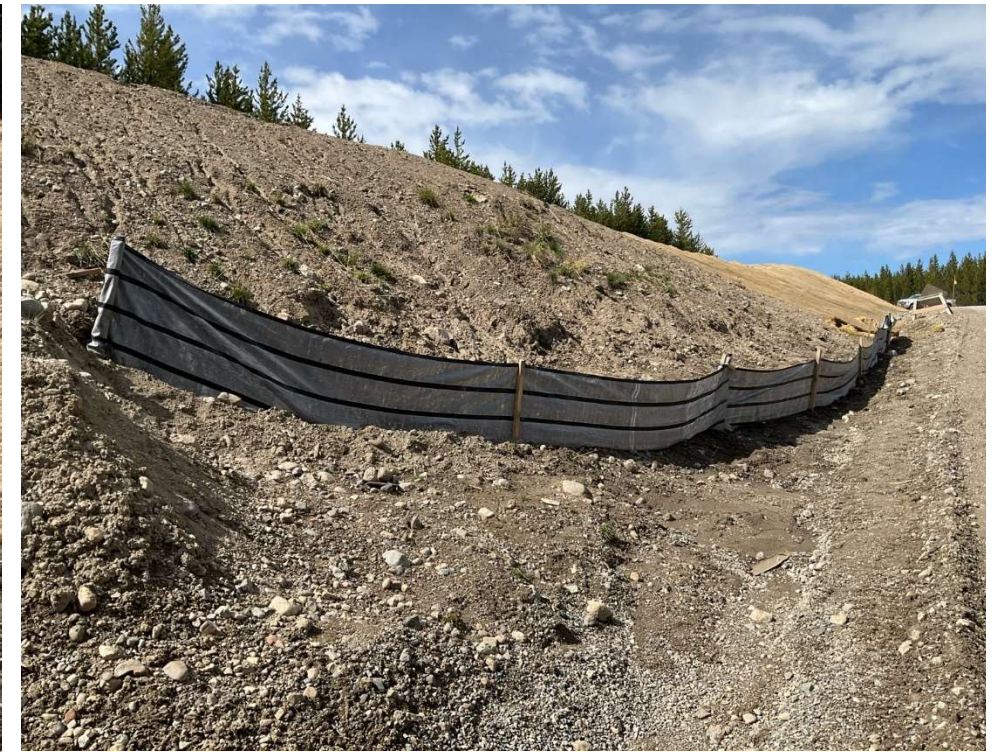
Photo 113696-3. Replacement sediment fencing installed on the slope along the C-Trail Access Road on approach to Watercourse 686 crossing.
