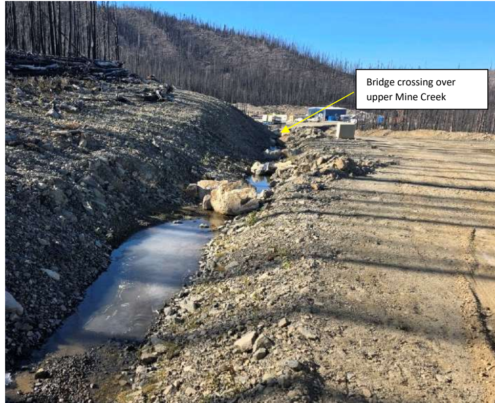
Photo 114456-1. Rock energy dissipaters installed within the ditch line along eastern approach to the bridge crossing over Mine Creek to the explosive magazine area.
