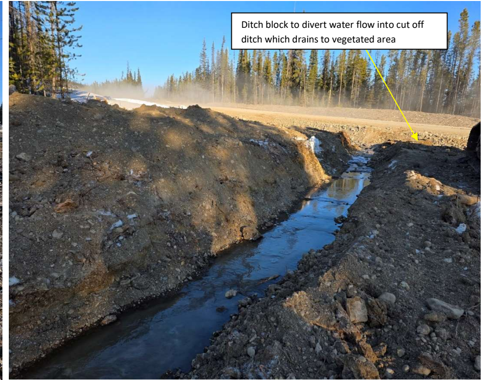
Photo 113513-3. Ditch block and cutoff ditch leading to vegetated area to prevent turbid water from draining into Watercourse 146. Photo taken morning of April 16, 2025.
