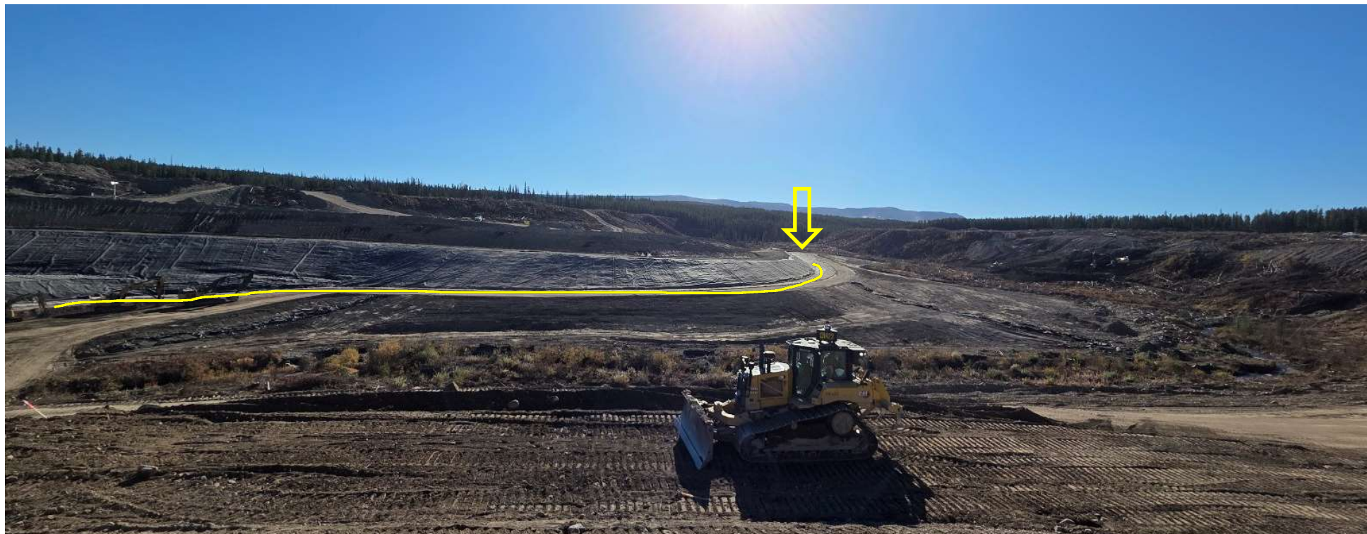
Photo 114458-3. Overview of the status of the Davidson Creek diversion channel construction within the Fresh Water Reservoir. Approximate pathway indicated on photo.
