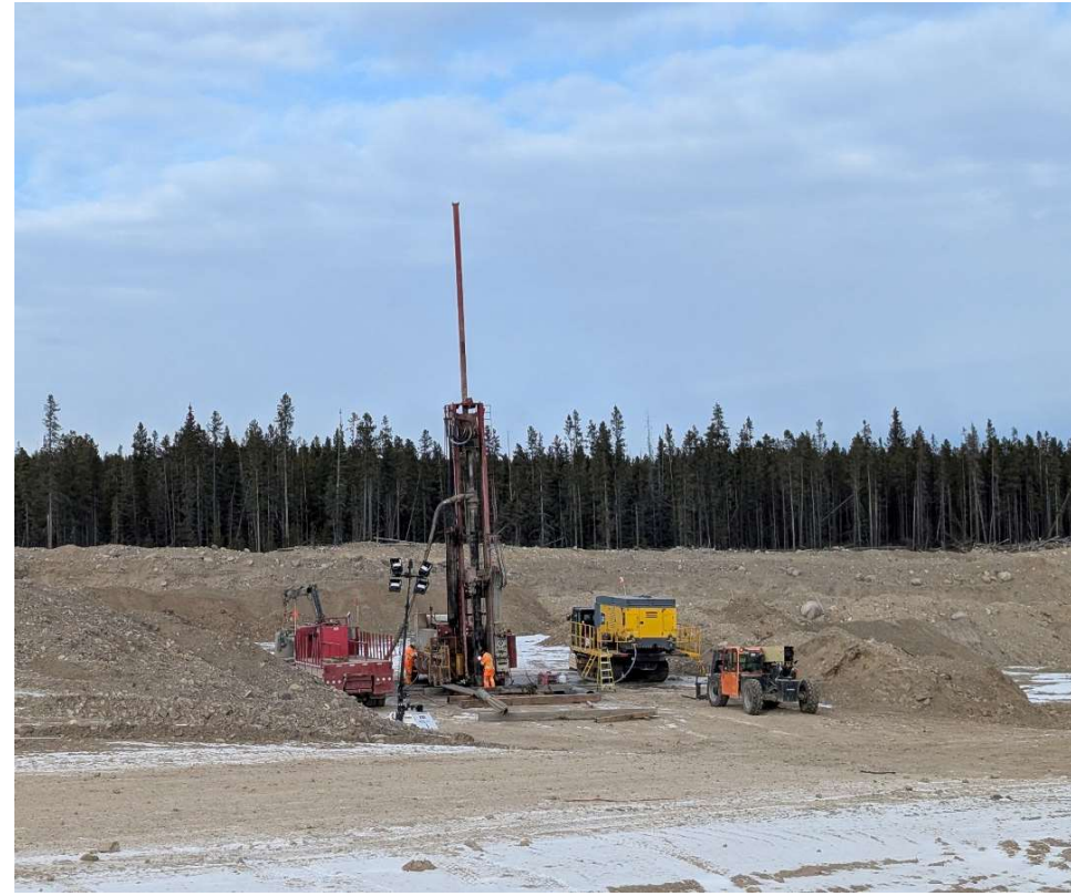
Photo 114711-1. One of the drill crews on-site installing monitoring and pumping groundwater wells. Drill rig in photo is located between the TSF and IECD.
