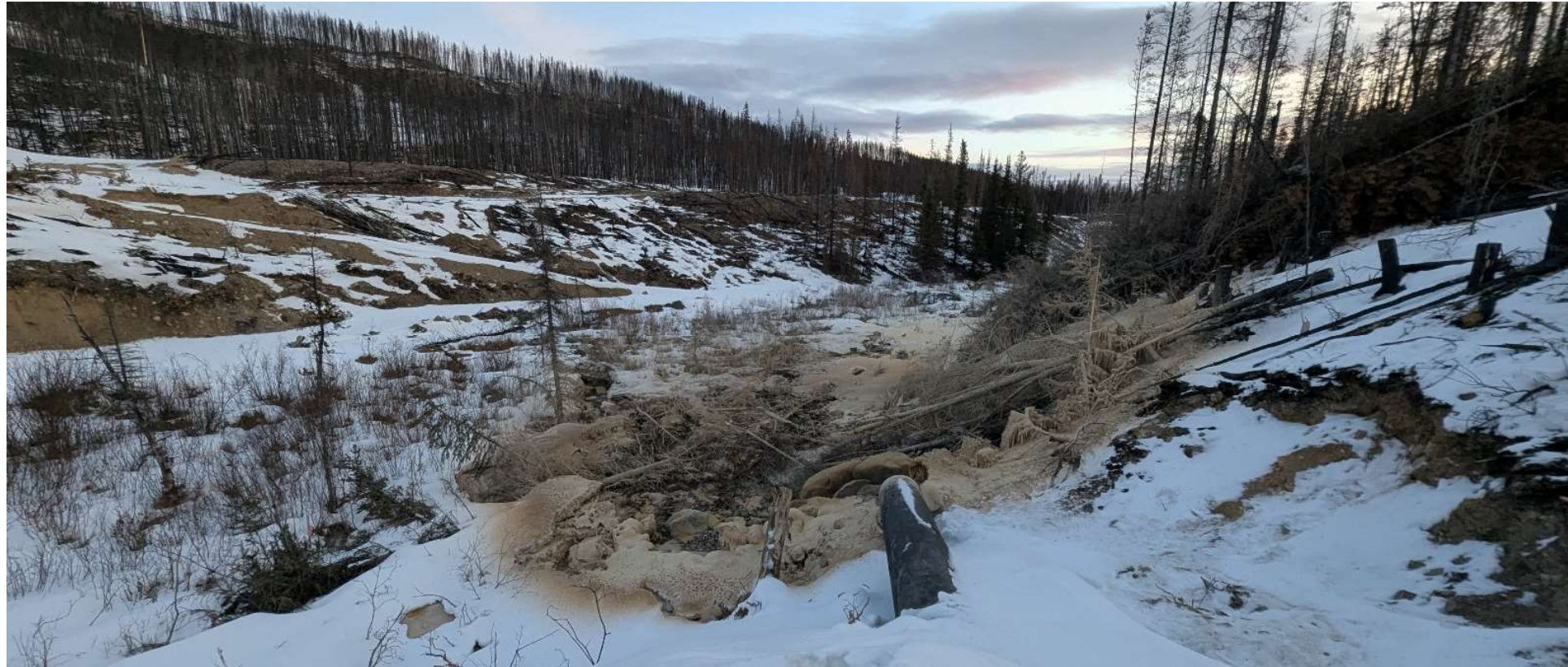
Photo 112943-1. Discharge point from pipeline delivering tailings from the Plant site into the Tailings Storage Facility (located downstream of the Central Water Transfer Pond).
