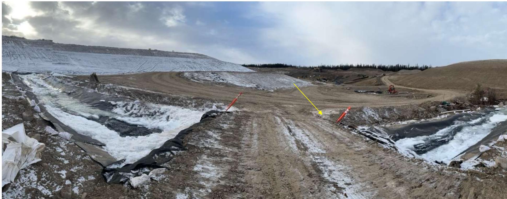
Photo 114703-8. Low spot identified as potential entry point for road runoff to enter into the Davidson Creek diversion channel within the Fresh Water Reservoir. Observation provided to BWG as an opportunity for improvement.
