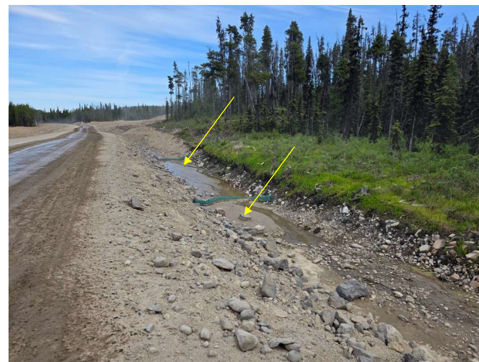
Photo 114077-3. Example of location along access road to Operations Camp where sediment accumulation has occurred within check dams. Examples also noted at other locations not included in photograph.
