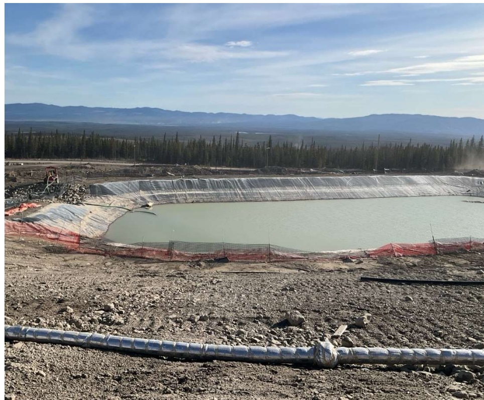
Photo 113700-1. Plant Site sediment control pond. The IEM team understands water being captured within this pond (impacted by PAG dust material at the Plant Site) is being used as process water and not being discharged to the environment.
