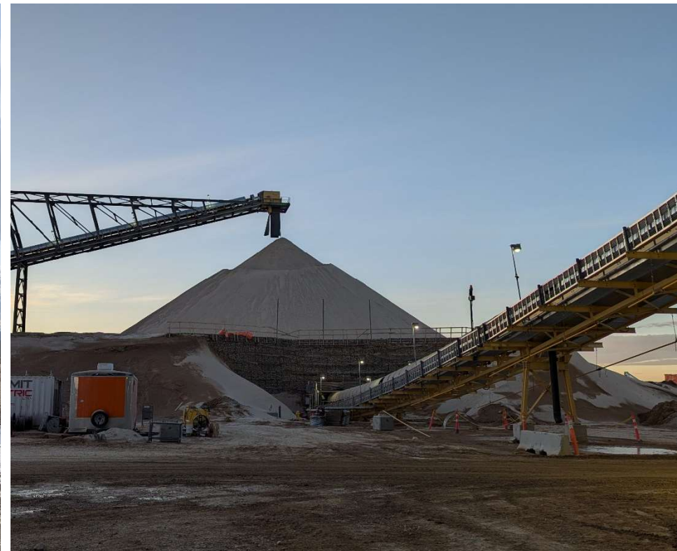
Photo 112941-3. Stockpile of high-grade ore at terminus of crusher/conveyor ready to be brought into plant site.
