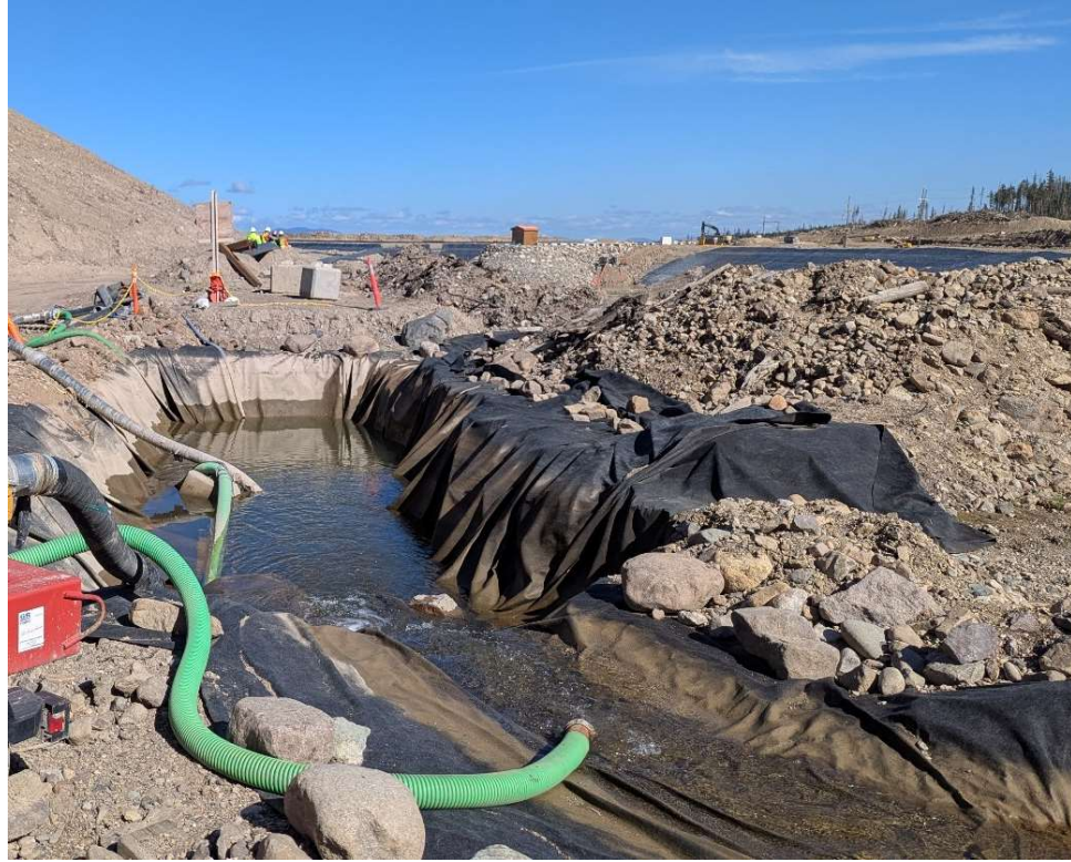
Photo 114314-2. Collection point for water from Mine Creek prior to entry into the WMP. Water is being pumped to CWTP via the South Collection Channel.
