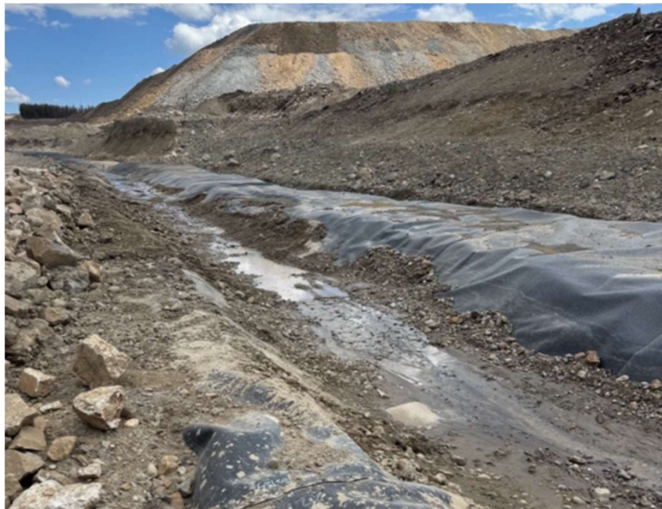
Photo 17. Confirmation material was removed from the PAG contact water ditch line adjacent to the Low-Grade Ore Stockpile. Photograph provided by BWG on July 28, 2025.
