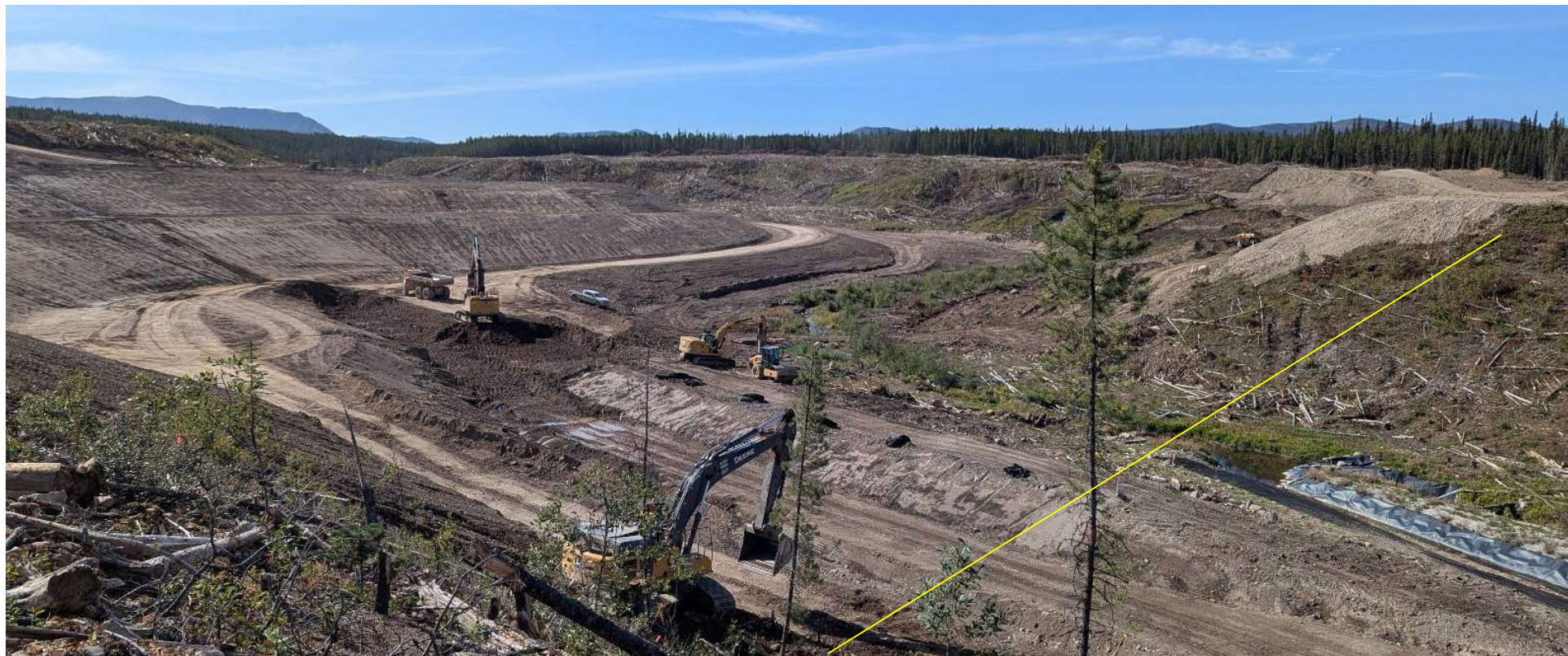
Photo 114317-7. Overview of crews working within the FWR. Approximate centerline of future dam indicated on photo.
