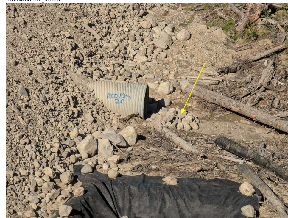
Photo 114319-1. Rock placed at outlet of culvert at Watercourse 636 at crossing along C-Trail Access Road (kilometer 9.5).
