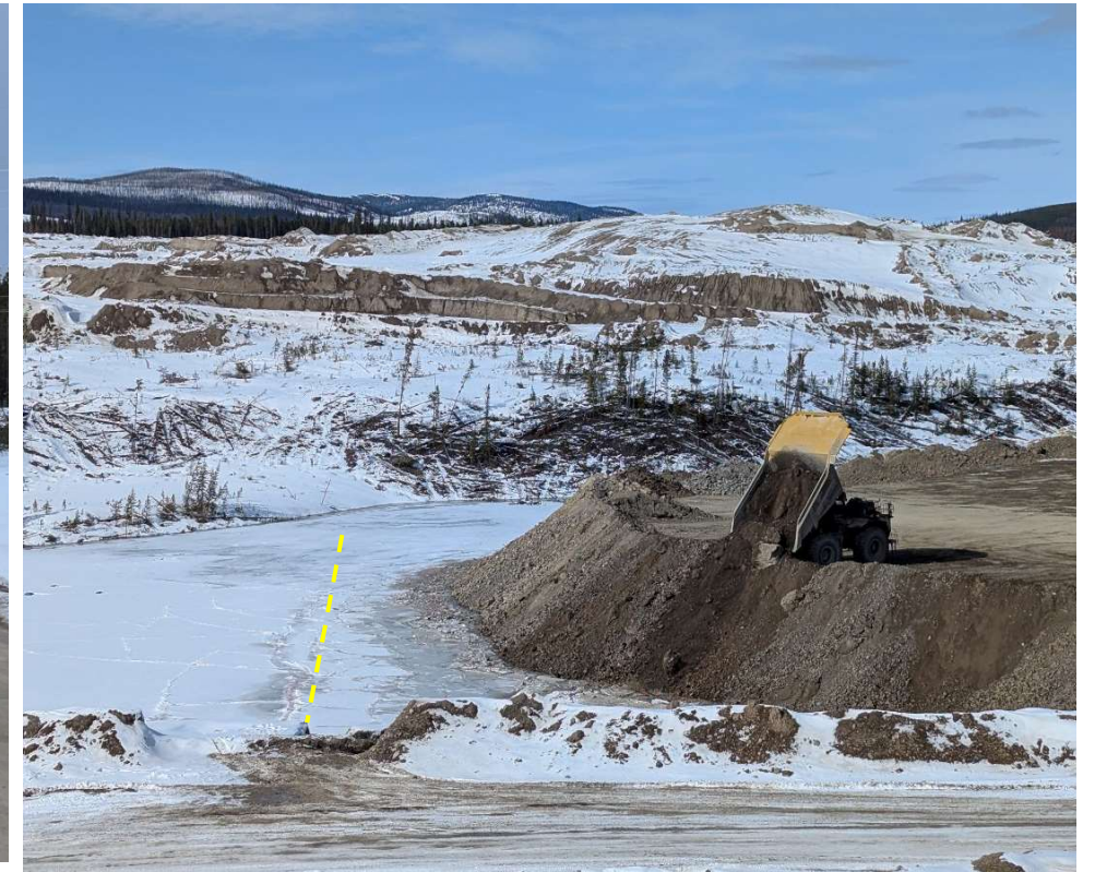
Photo 113330-1. PAG material being placed at the PAG Dump. Approximate centerline of former Davidson Creek Diversion Structure (now under water) indicated on photo.
