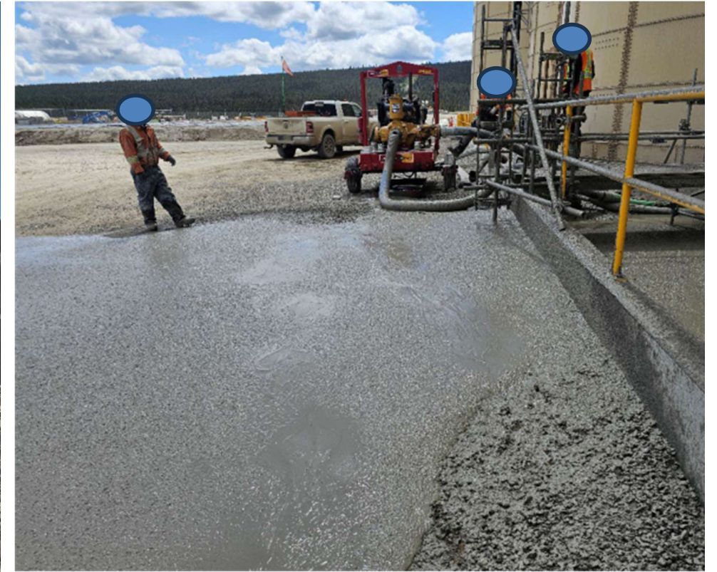
Photo 2. Spill of processing slurry that occurred on July 3, 2025, at the Plant Site. Photograph from end of spill report to ENV provided by BWG to IEM team on August 13, 2025.
