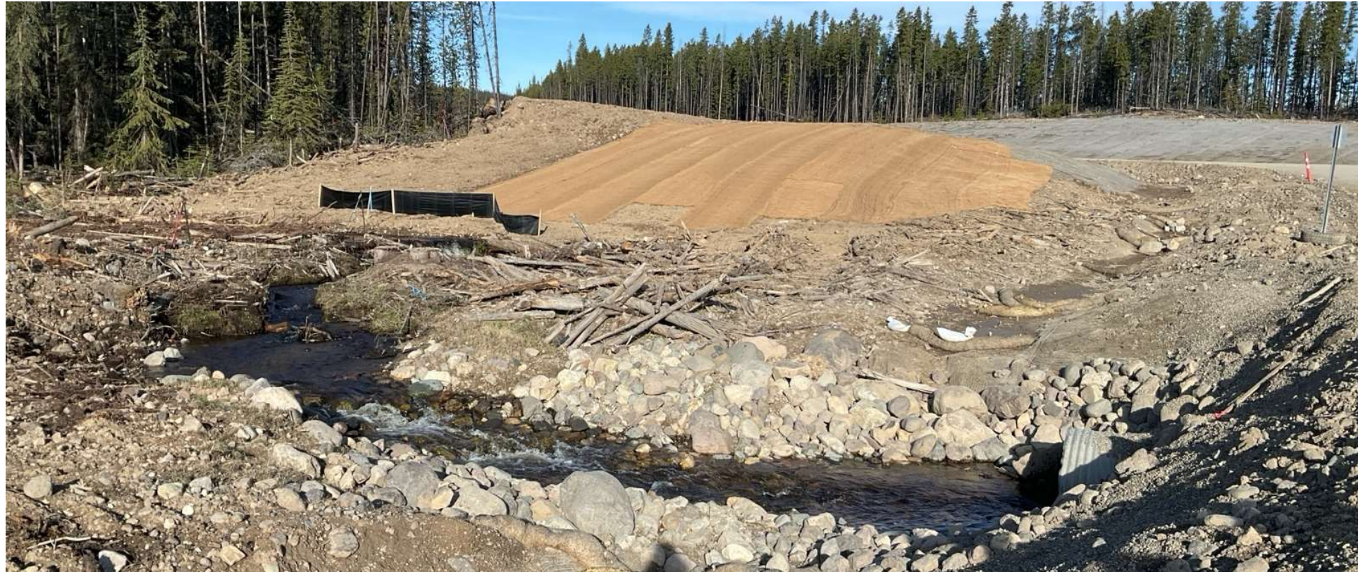
Photo 113699-1. Overview of Watercourse 146 crossing (on access road to Operations Camp). Water observed to be running clear at time of visit. Recently installed ESC measures (sediment fencing and erosion control blankets) also noted.
