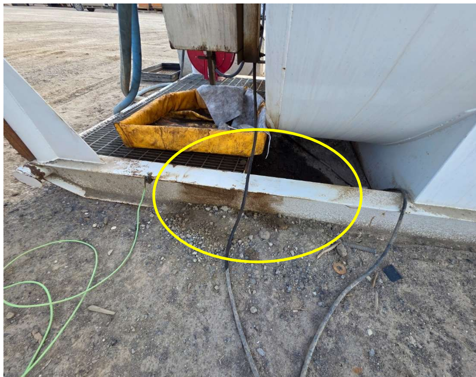
Photo 114080-1. Hydrocarbon spill to ground beneath fuel tank staged at the Andrew's Hill laydown.
