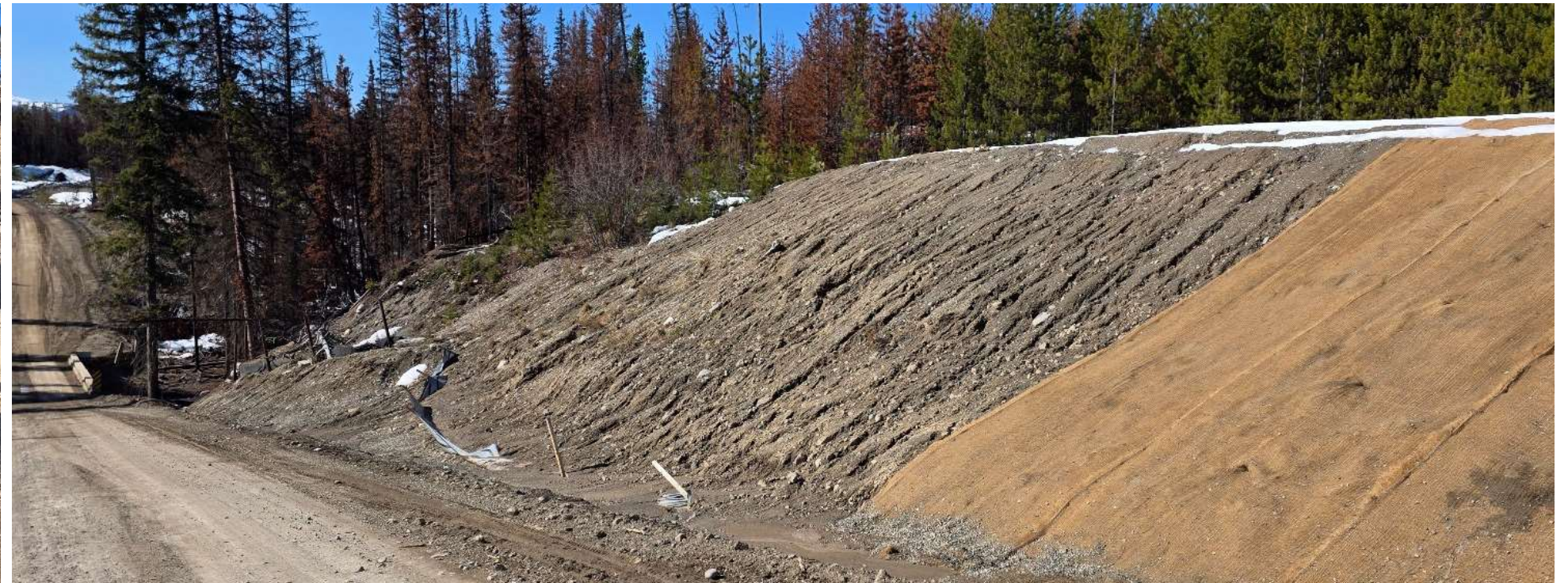
Photo 113555-9. Overview of slope above Watercourse 636 crossing where ESC measures will likely soon require maintenance/repair in order to minimize sediment transport to Watercourse 636. IEM will complete a follow up visit to this location to observe area in a future visit.
