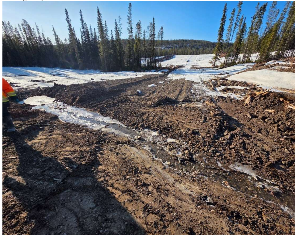
Photo 113513-4. Terminus of cutoff ditch (see photo 113513-3) installed to prevent turbid water from draining into Watercourse 146 along the access road to Operations Camp. Photo taken morning of April 16, 2025.
