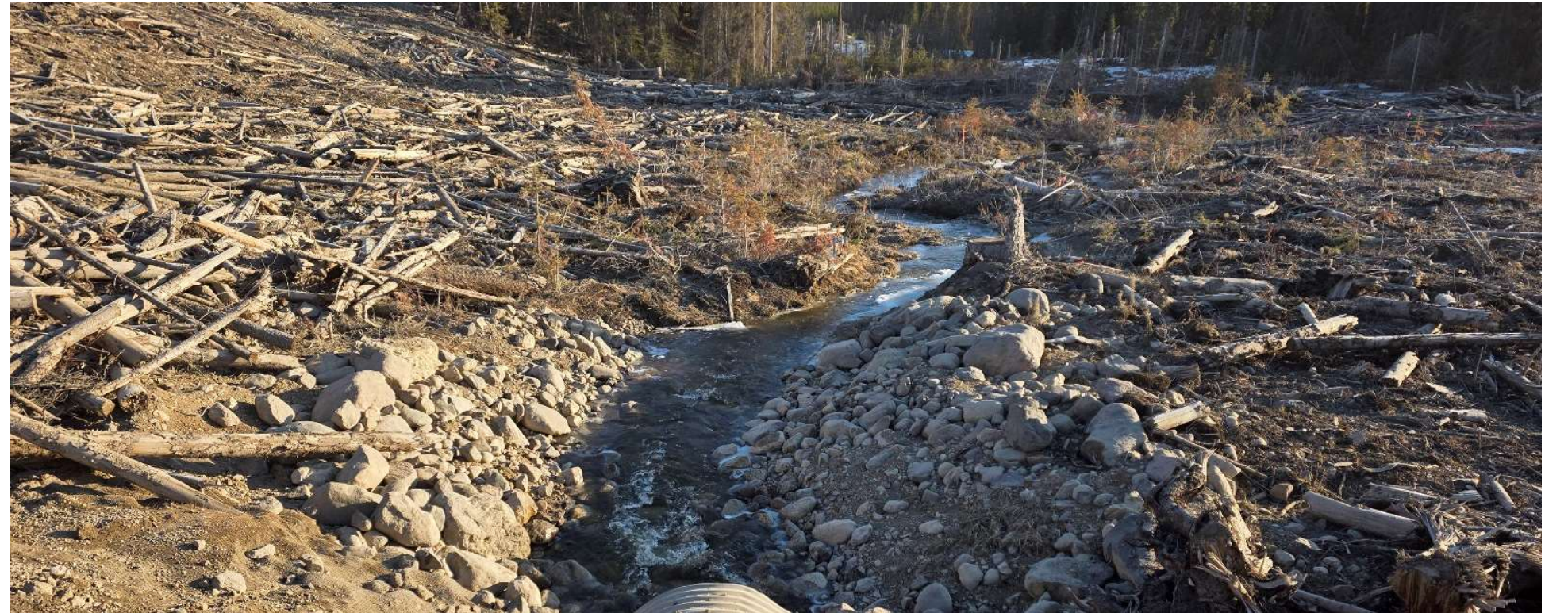
Photo 113513-5. Overview of flow in Watercourse 146 following the installation of upstream ditch block to divert turbid water flow. Photo taken morning of April 16, 2025.
