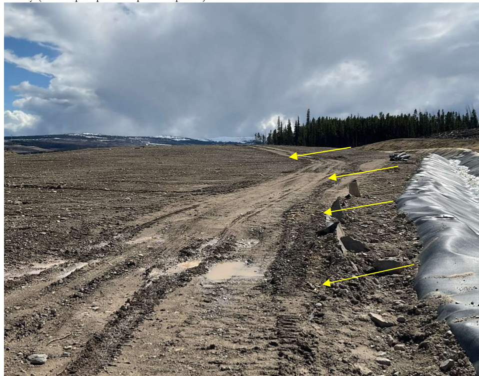
Photo 113690-1. Overview of area adjacent to the NDC following contouring to prevent water from running into ditch line. Direction of grading indicated on photo.
