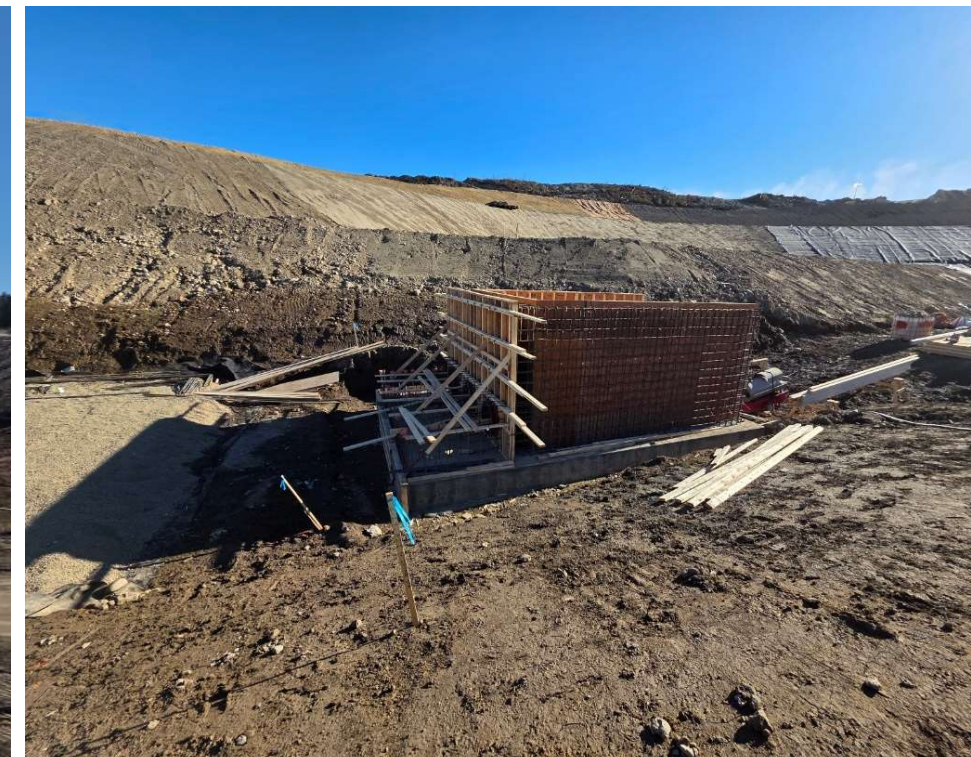
Photo 114458-11. Formwork for a portion of the concrete flow chamber structure being constructed within the Fresh Water Reservoir.
