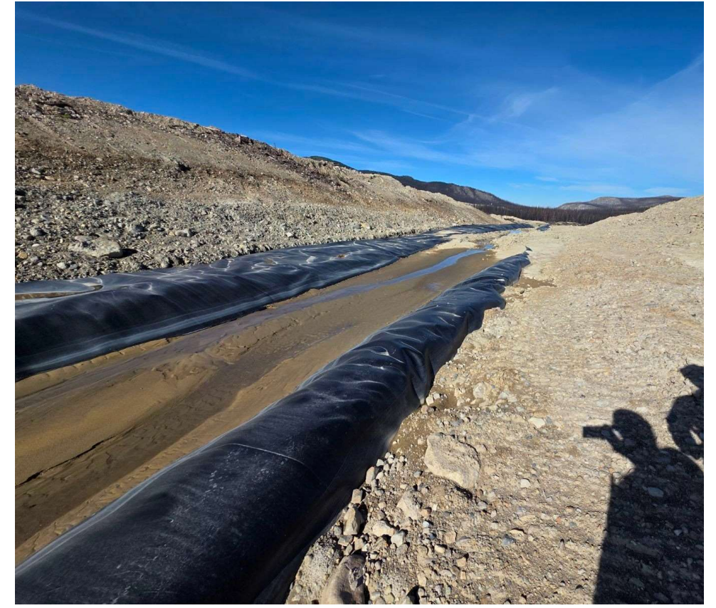
Photo 114083-2. Excess sediment accumulation within the lined PAG contact water ditch line adjacent to the Low-Grade Ore stockpile.
