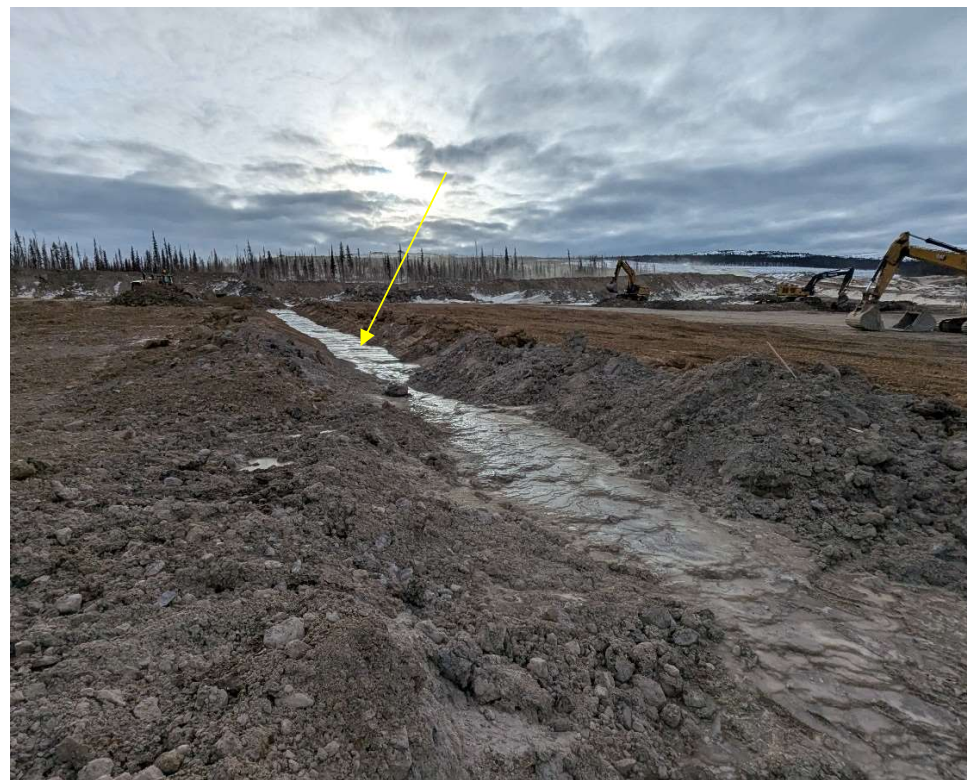
Photo 112953-5. Ongoing construction of the drainage channels beneath the future LGO stockpile pad.
