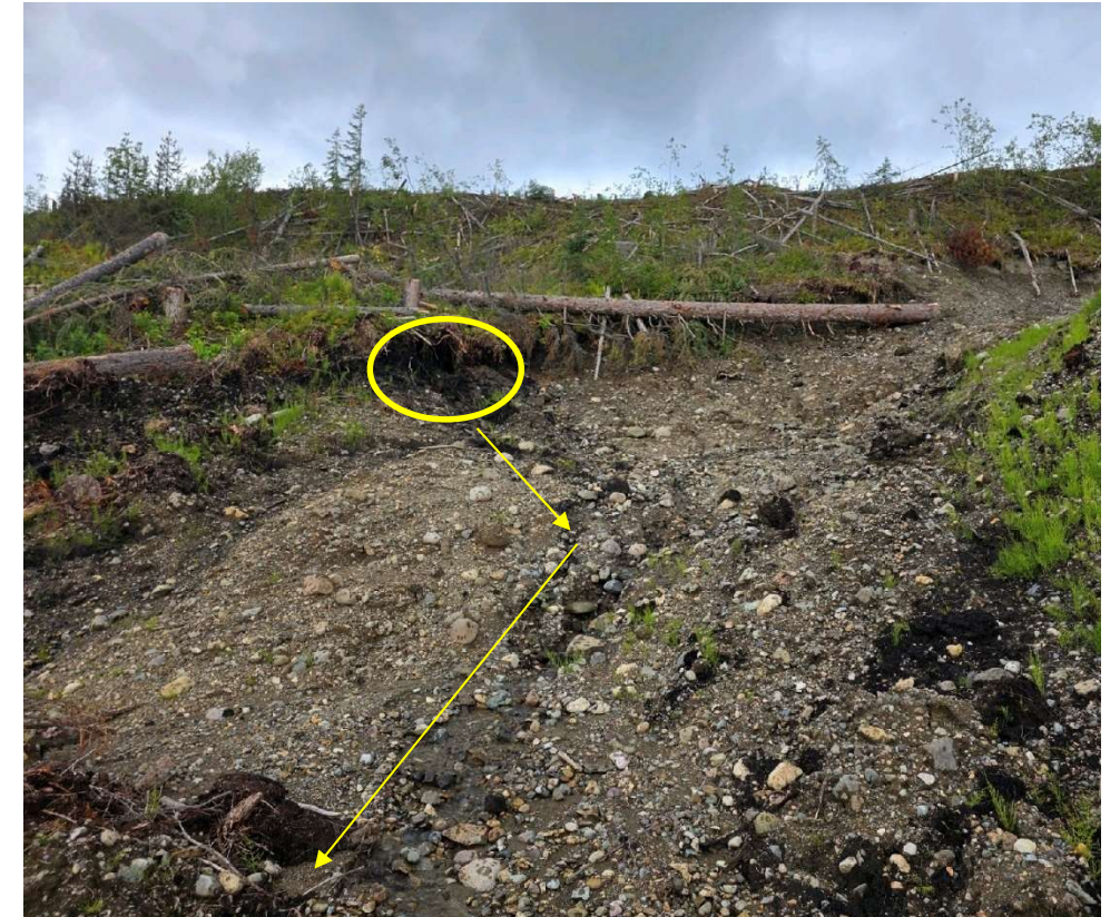
Photo 114201-6. Seep coming from footprint of former slide area into Davidson Creek within the Fresh Water Reservoir worksite.
