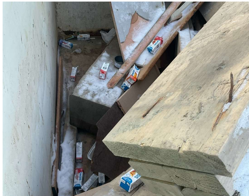
Photo 114731-1. Food/domestic waste observed in an open top bin staged at the Andrew's Hill laydown. BWG confirmed bin containing these contents had been removed and replaced with an empty one on December 4, 2025.
