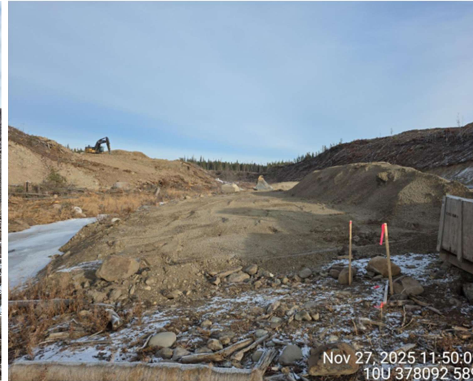
Photo 20. Stockpile of aggregate pulled back from edge of Davidson Creek downstream of the Fresh Water Reservoir. Photograph provided by BWG on December 4, 2025.
