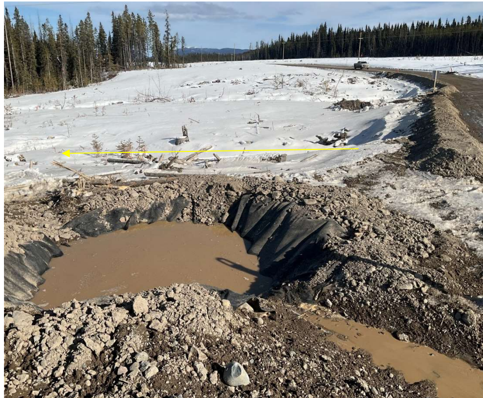
Photo 113343-1. Turbid water accumulated within the sump installed adjacent to Watercourse 146 on the access road to the Operations Camp. Approximate pathway of watercourse indicated on photo.
