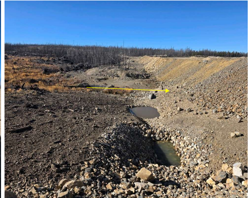
Photo 114457-2. Improvements to drainage (collection sumps, rock armoring) in drainage adjacent to the road crossing of Mine Creek downslope of the LGO stockpile pond. Mine Creek flow indicated on photo.
