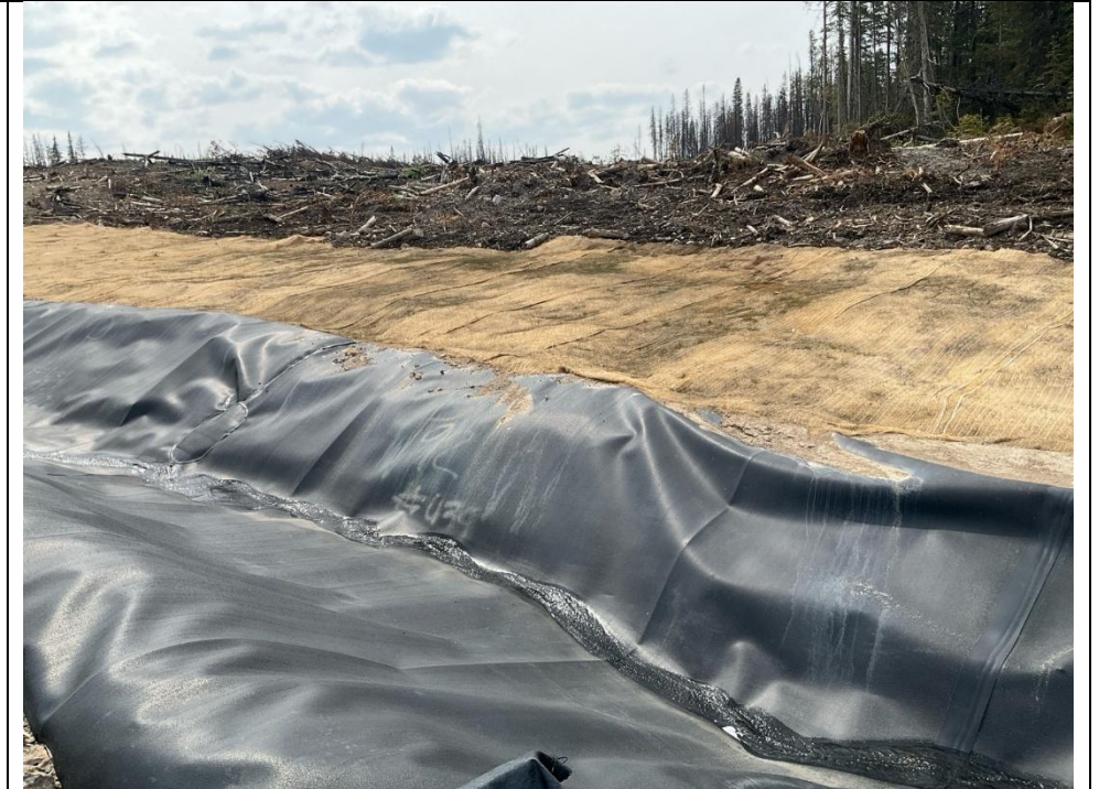
Photo 113870-1 Vegetation has started to grow through the erosion control matting at the Northern Diversion Channel.
