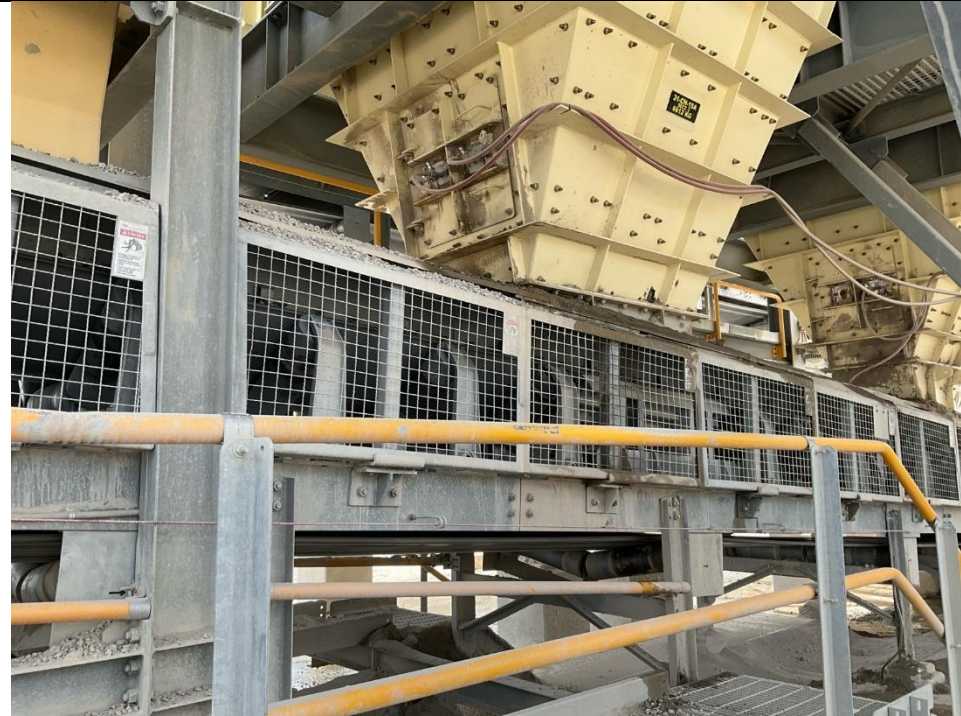
Photo 113867-3 Spray point at the tertiary crusher.
