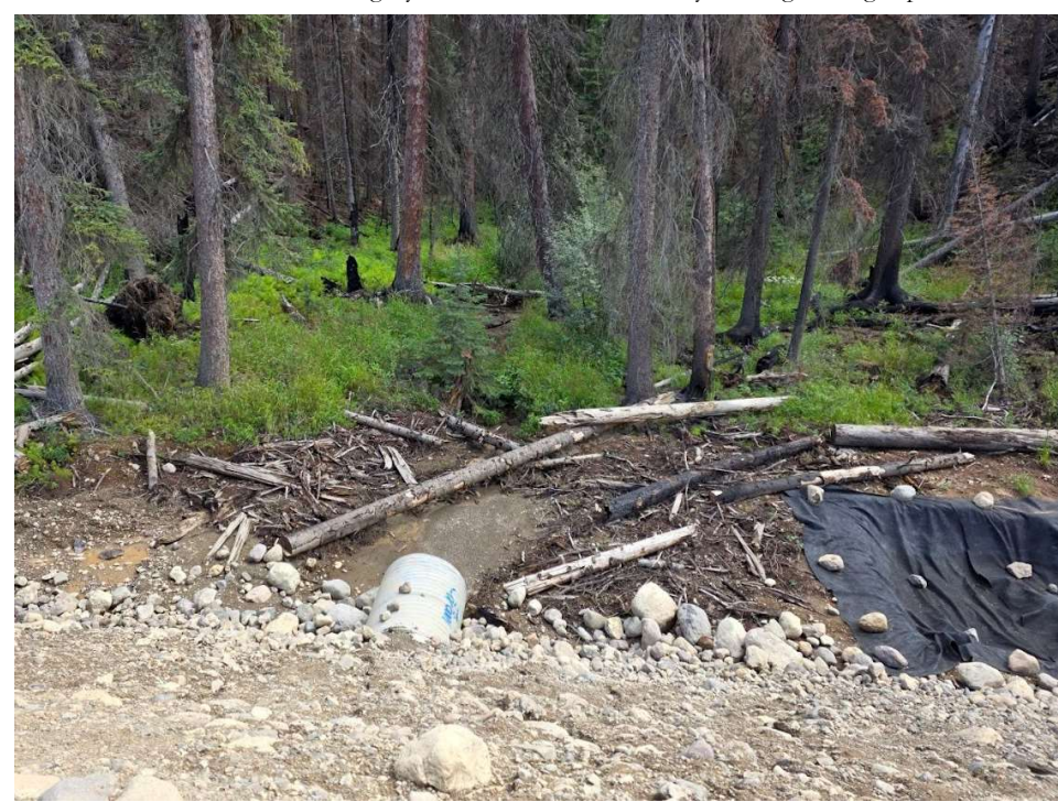
Photo 114199-2. Lack of energy dissipation on downstream side of Watercourse 636 culvert crossing at 9.5 km on the C-trail access road.
