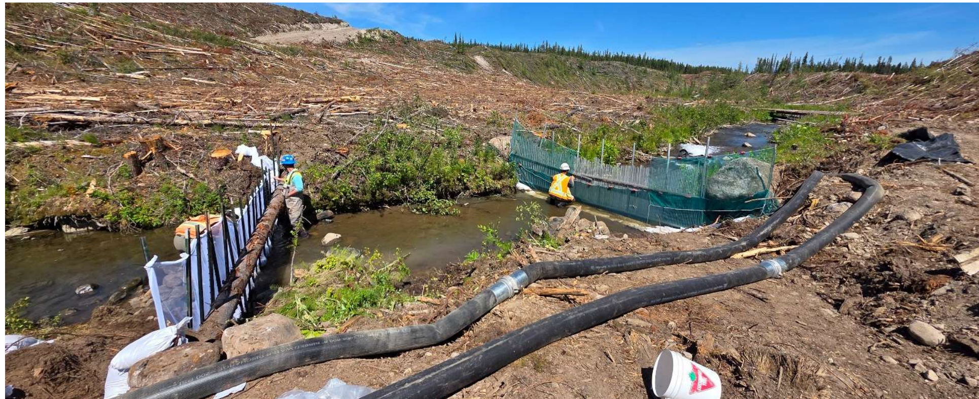
Photo 114069-5. Crews working on establishing fish barriers on Davidson Creek within the cleared footprint of the Fresh Water Reservoir.
