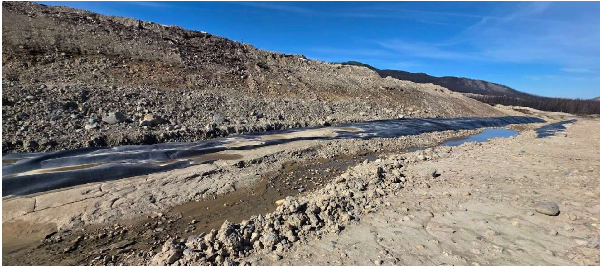
Photo 114083-1. Excess sediment accumulation (along with what appears to be fill material from the nearby pad) within the lined PAG contact water ditch line adjacent to the Low-Grade Ore stockpile.
