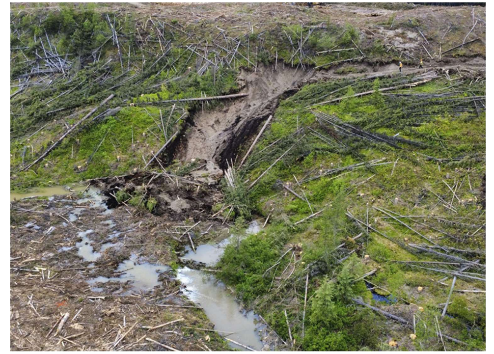
Photo 19. Slide into Davidson Creek (above the DC-05 compliance sampling point) within the Fresh Water Reservoir clearing worksite. Photograph provided by BWG on July 27, 2025.
