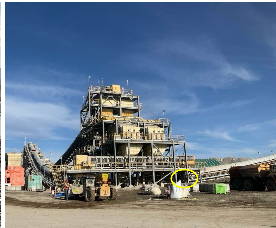
Photo 113701-1. Location on the crusher conveyor system where water is sprayed onto high grade ore prior to being stockpiled at the Plant Site.
