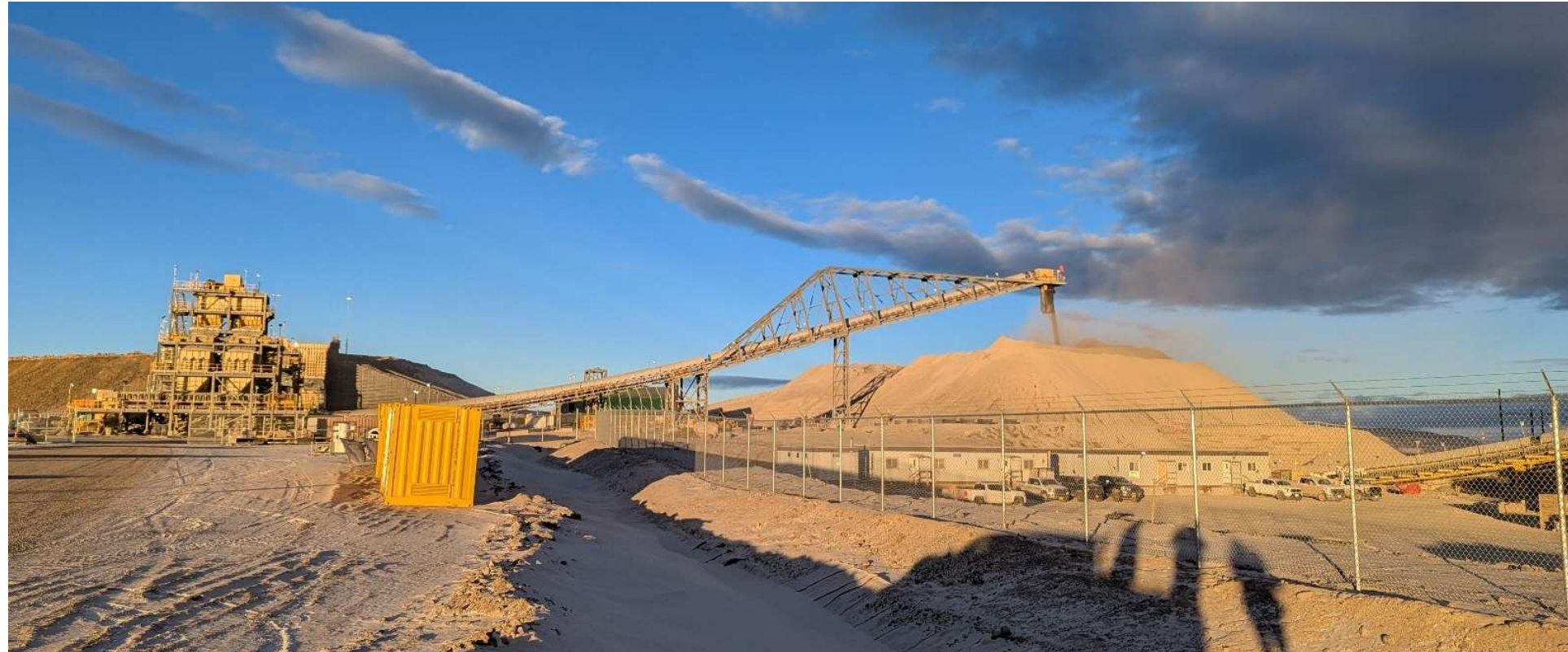
Photo 114727-1. Overview of the conveyor drop point at the Plant Site. Material falling onto high grade ore stockpile appeared to be wetted at the time of observation.
