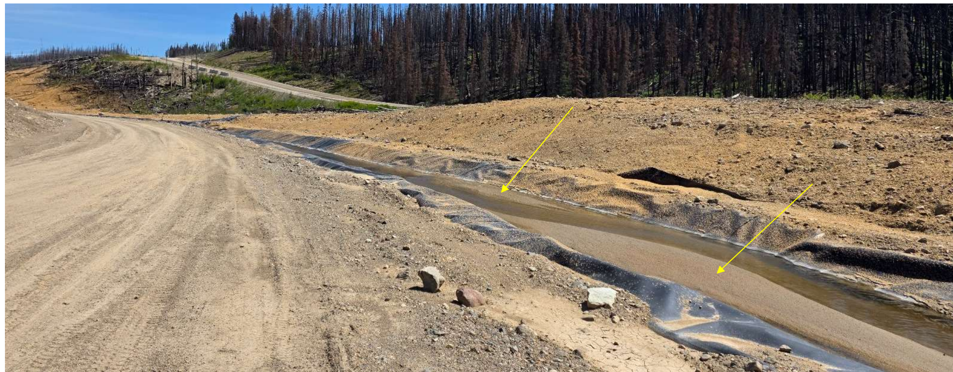
Photo 114078-3. Excess sediment accumulation within the lower extents of the Southern Collection Channel near its discharge point into the Central Water Transfer Pond.
