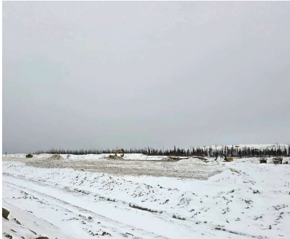
Photo 113125-2. Crews continue placement of 'zone s' till liner along the base of the LGO stockpile pad.
