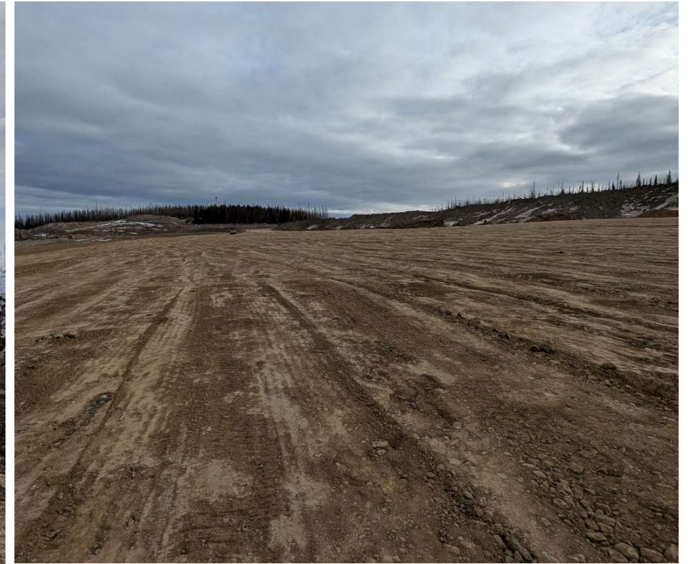
Photo 112953-7. Overview of preparation of the compacted till liner under construction at the LGO stockpile pad.
