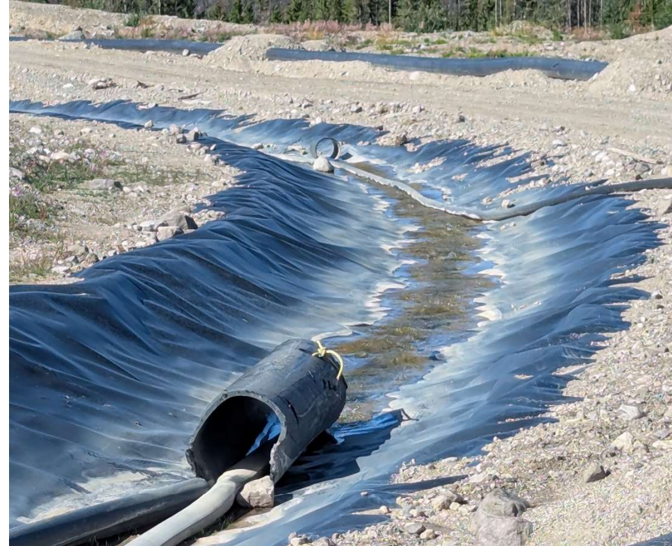
Photo 114314-5. Discharge point of water from the Mine Creek Diversion (prior to entering WMP) into the South Collection Channel (ultimately leads to the CWTP).
