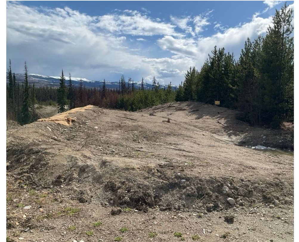
Photo 113696-2. Grading to direct water away from the slope adjacent to the C-Trail Access road crossing of watercourse 686 (km 9.5 bridge).
