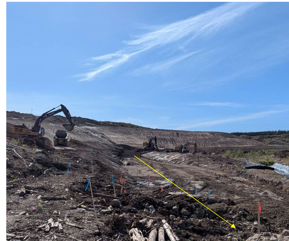
Photo 114317-1. Works on the floor of the FWR to develop the future diversion channel and concrete flow chamber structure to facilitate water passage through the site during construction, and ultimately IFNs to Davidson Creek from downstream side of dam once complete. Flow direction indicated on photo.
