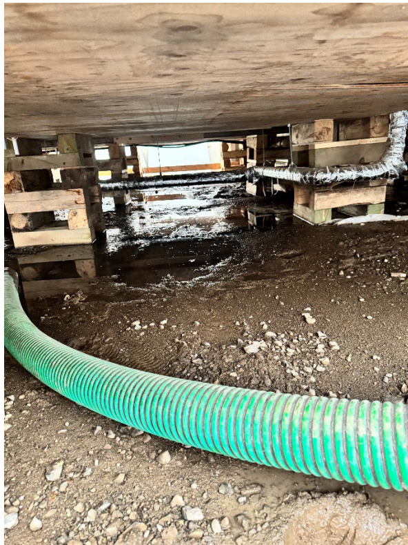
Photo 5: Spill Clean Up
