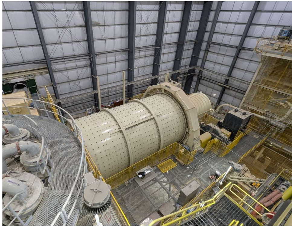
Photo 112941-4. Overview of components inside of plant site building currently undergoing commissioning.
