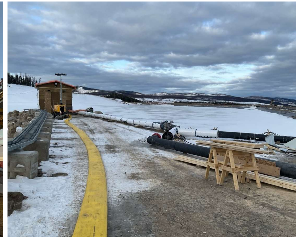
Photo 112947-4. Status of decant tower at the water management pond. Water temporarily being pumped to plant site via hose until permanent pipelines can be implemented.
