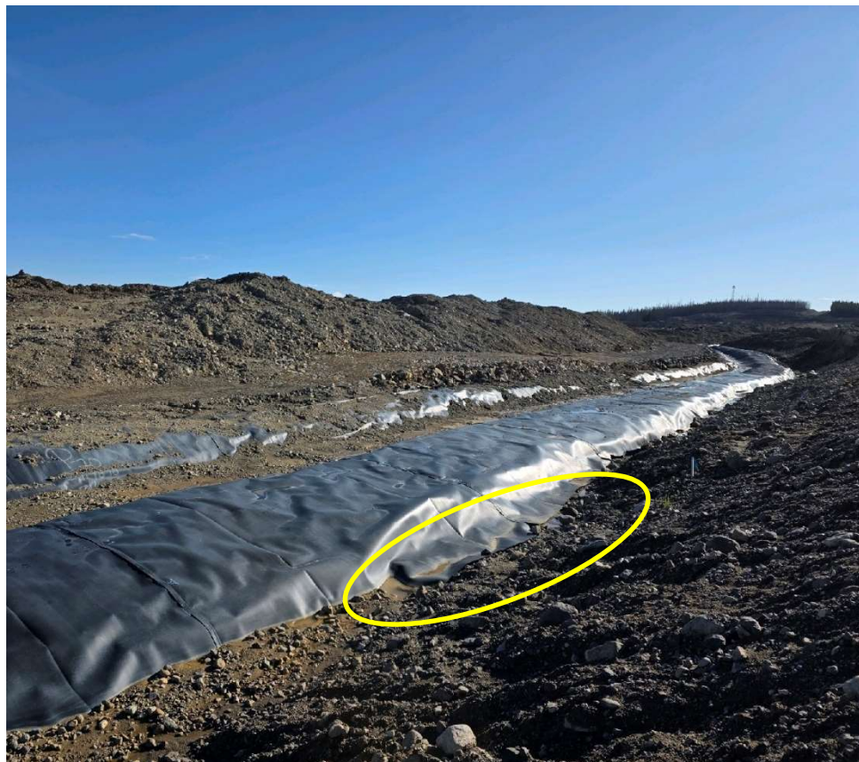
Photo 114219-2. Example location along LGO stockpile ditch line where liner is raised (not keyed in) and allowing water to flow beneath it.
