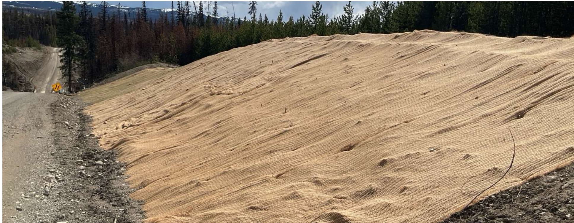
Photo 113696-5. Overview of additional erosion and sediment control blankets placed on slope along the C-Trail Access Road on approach to Watercourse 686 crossing.
