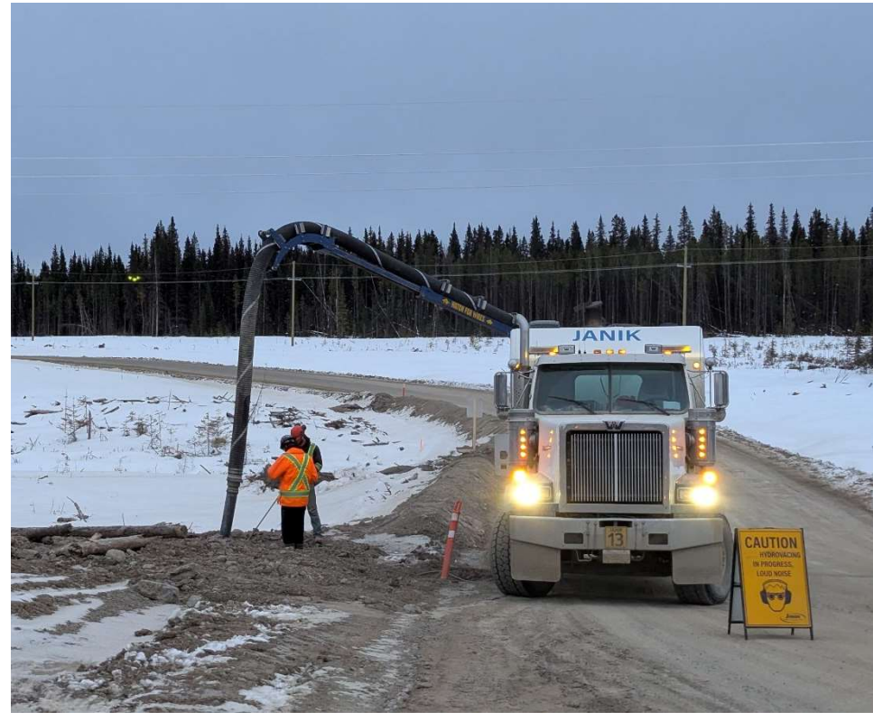
Photo 113345-3. Crews removing turbid water accumulation in sump adjacent to Watercourse 146 (as seen in photo 113343-1) to prevent overtopping.
