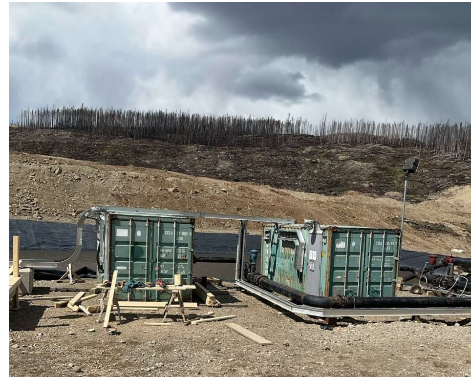
Photo 113688-2. Electric pump units installed at the CWTP to discharge water to Davidson Creek.
