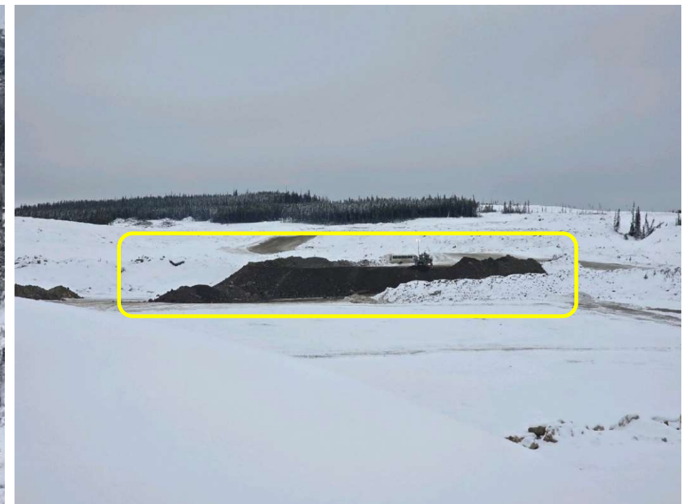
Photo 113132-1. Crews placing material at the 'PAG dump' immediately upstream of the TSF dam.
