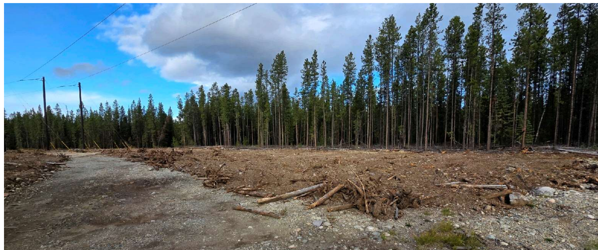
Photo 114490-5. Overview of the reclamation works at 119.5km on the Kluskus Forest Service Road.
