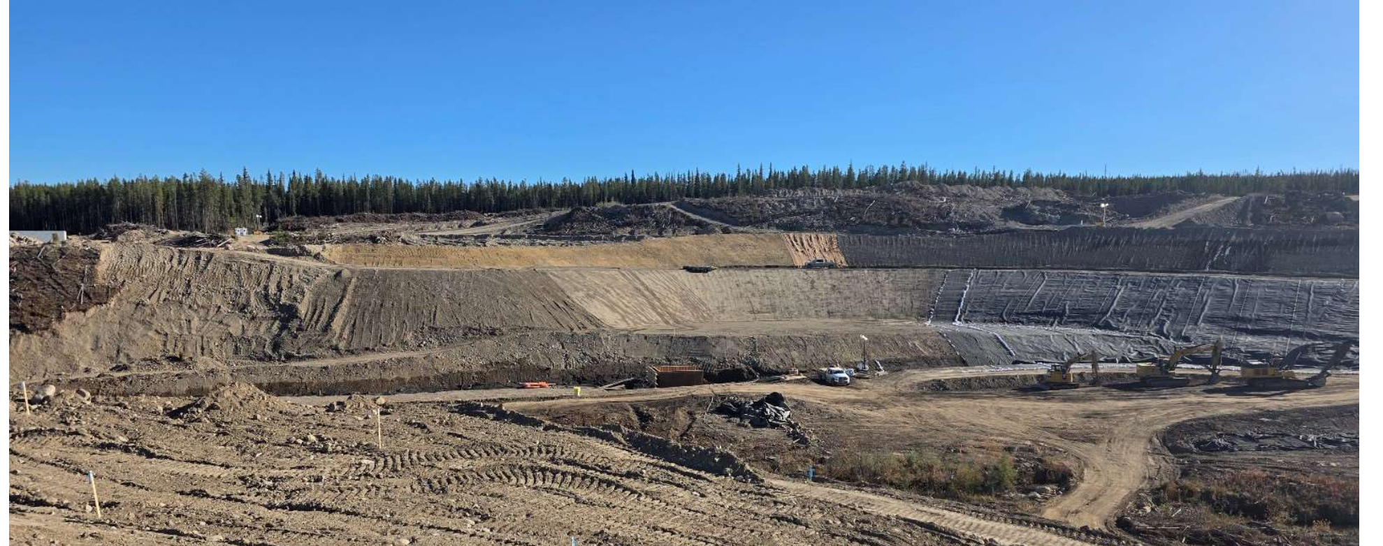
Photo 114458-2. Liner installation continues at the eastern end of the Fresh Water Reservoir.
