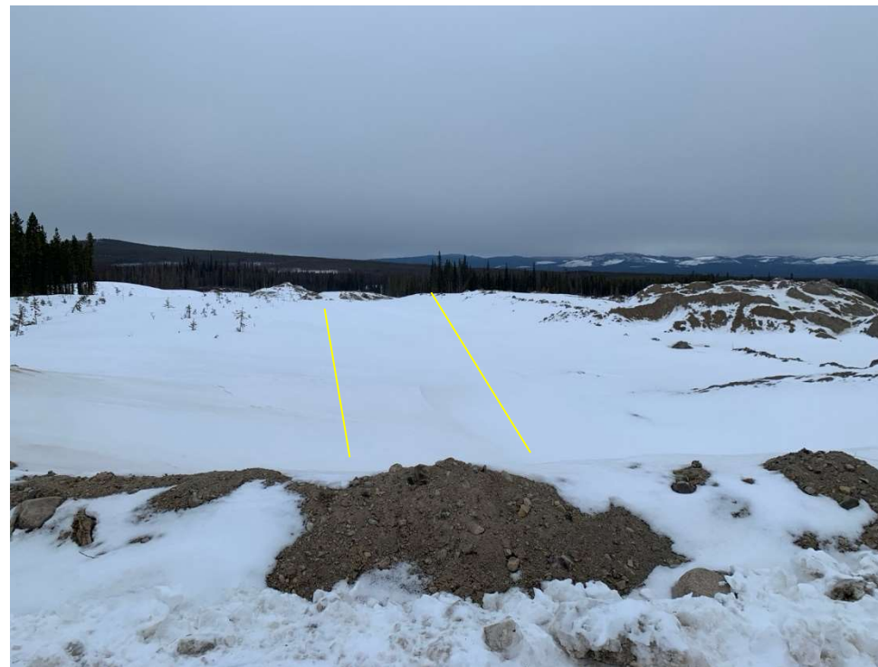
Photo 113351-2. Overview of snow filled north diversion ditch. Plowed access not available at time of visit due to recent snowfall, however BWG plan to re-establish access imminently.
