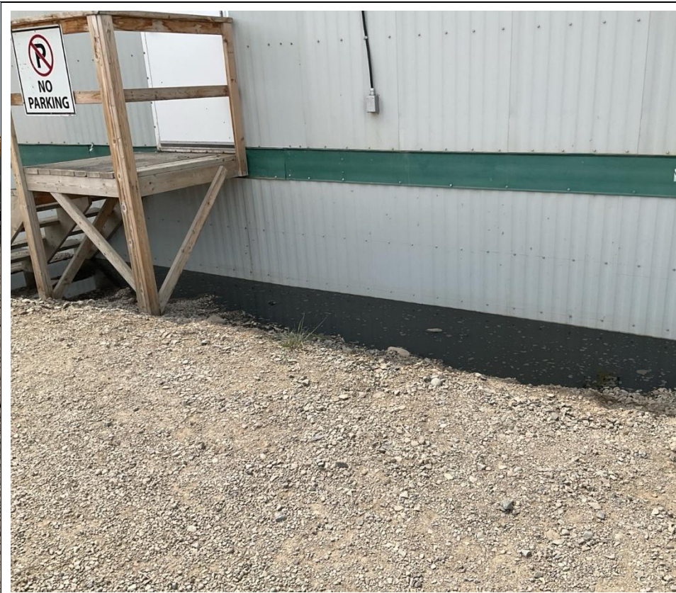
Photo 113868-1 Sewage leak below the bunk house at the Construction Camp.
