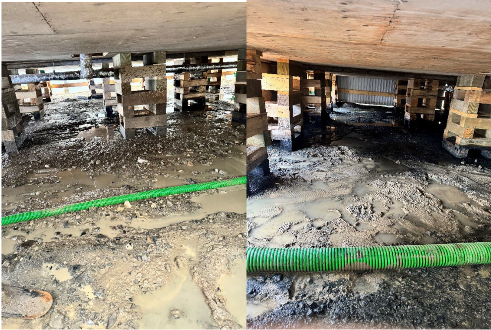
Photos 1 & 2: Spill Photos
