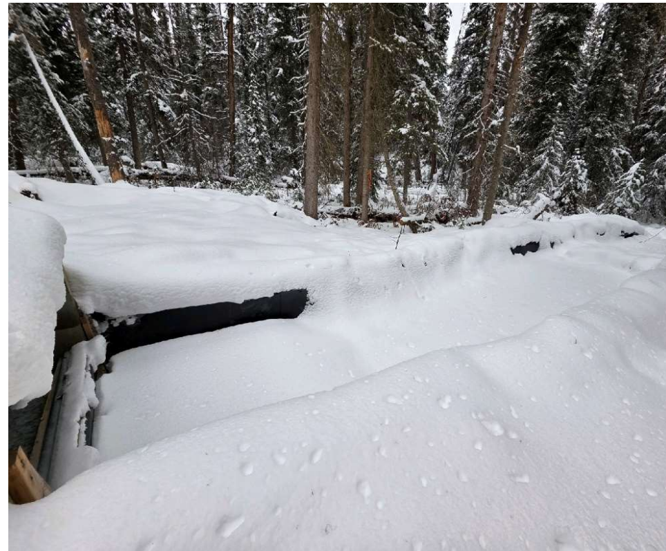
Photo 113127-1. WMP outfall structure (which discharges to Davidson Creek). Observed to not be operating at time of visit due to frozen pumps.
