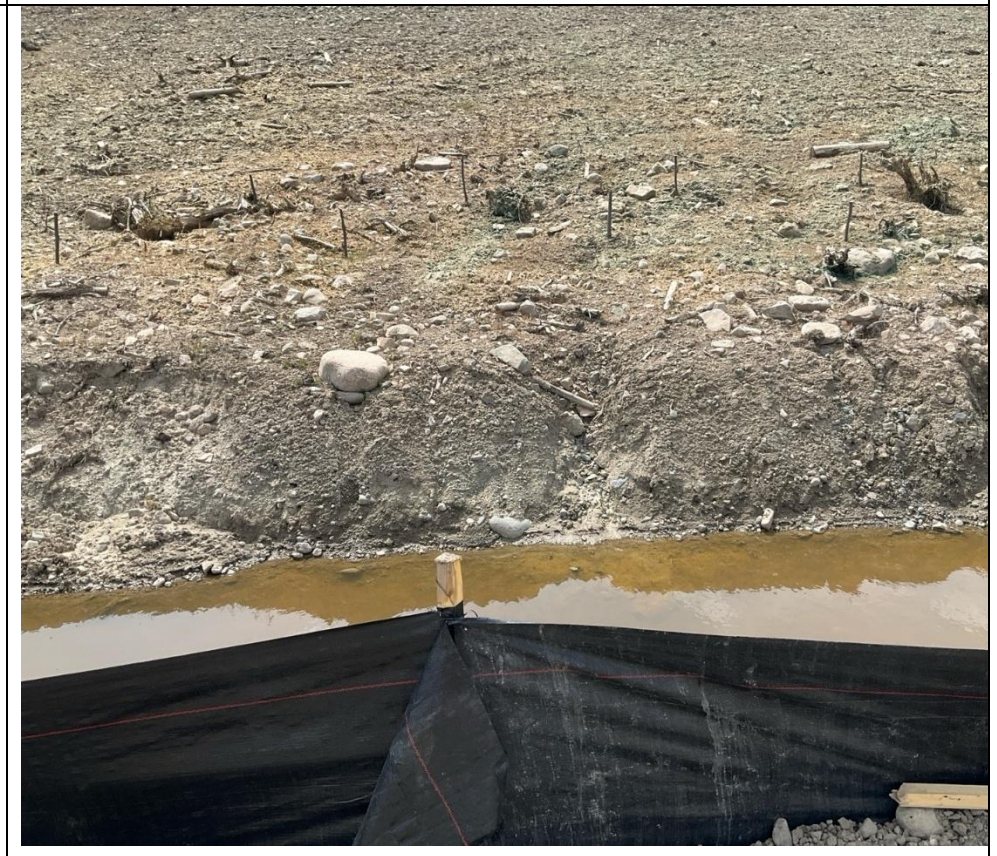
Photo 113866-1 Live willow staking, hydroseeding, and amphibian fence installed near the Operations Camp.
