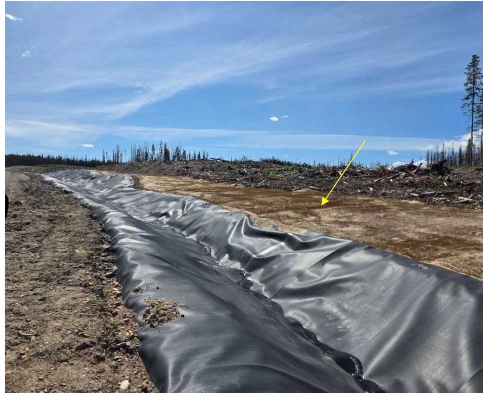
Photo 114073-5. Vegetation growth observed beneath the erosion and sediment control blankets installed on the high side of the North Diversion Channel.
