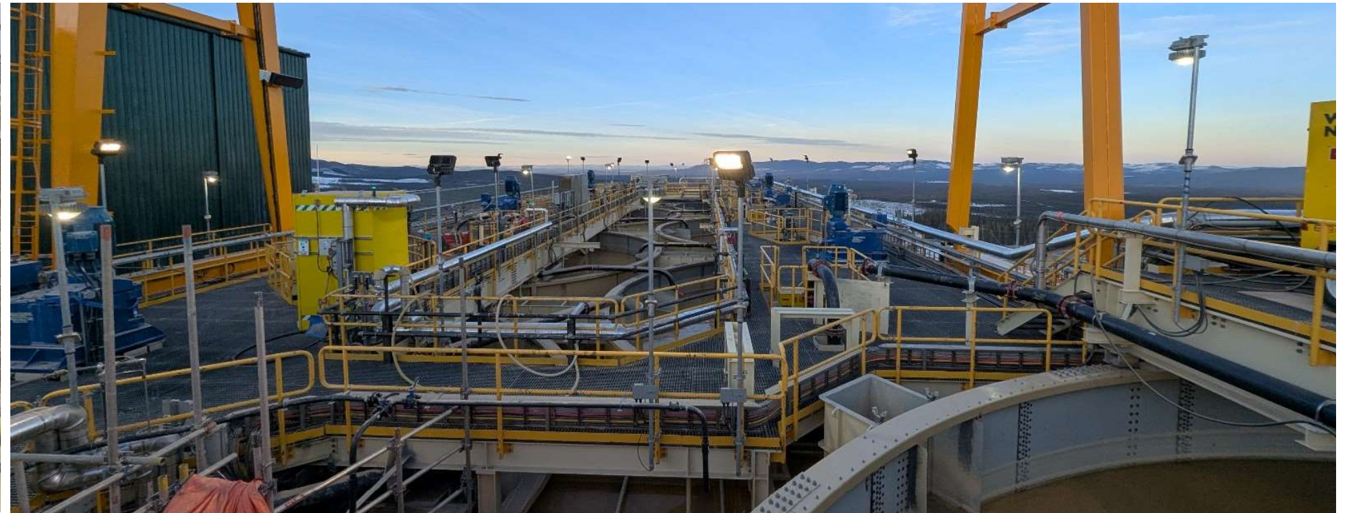
Photo 112941-9. Overview of leach circuit components currently undergoing commissioning.
