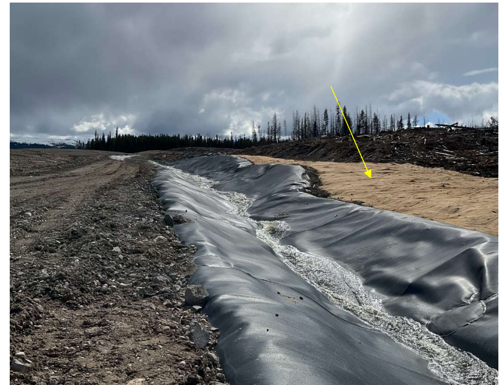
Photo 113691-4. Erosion control blankets installed along portion of high side of the NDC.
