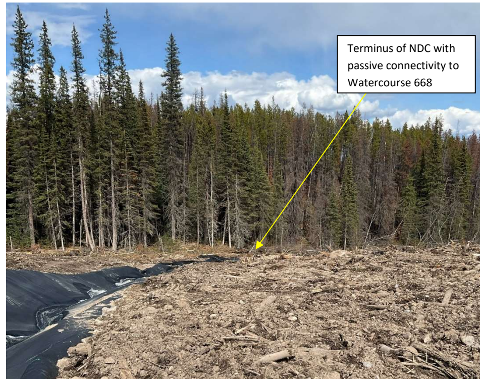
Photo 113691-3. Overview of the terminus of the NDC following application of topsoil and rough and loose surface application.
