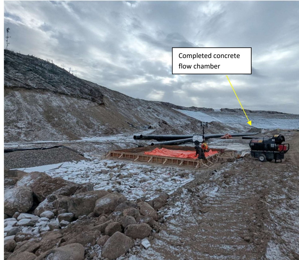
Photo 114705-3. Crews working on discharge channel downstream of the concrete flow chamber within the Fresh Water Reservoir.
