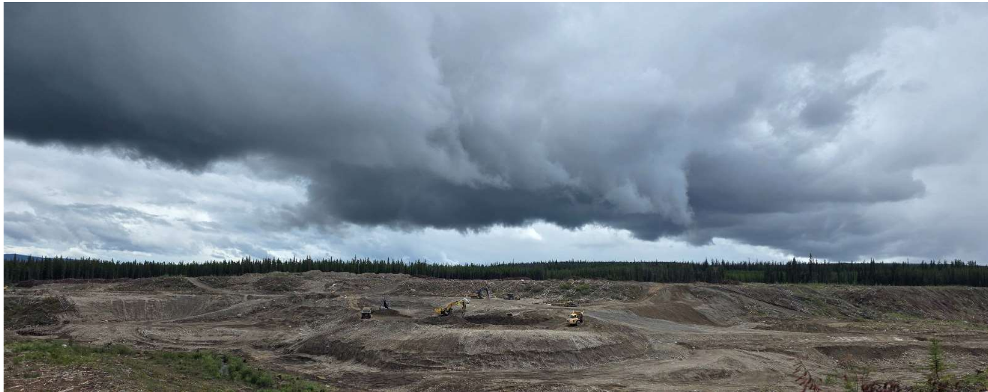
Photo 114202-5. Overview of crews working on excavation and shaping of the Fresh Water Reservoir.
