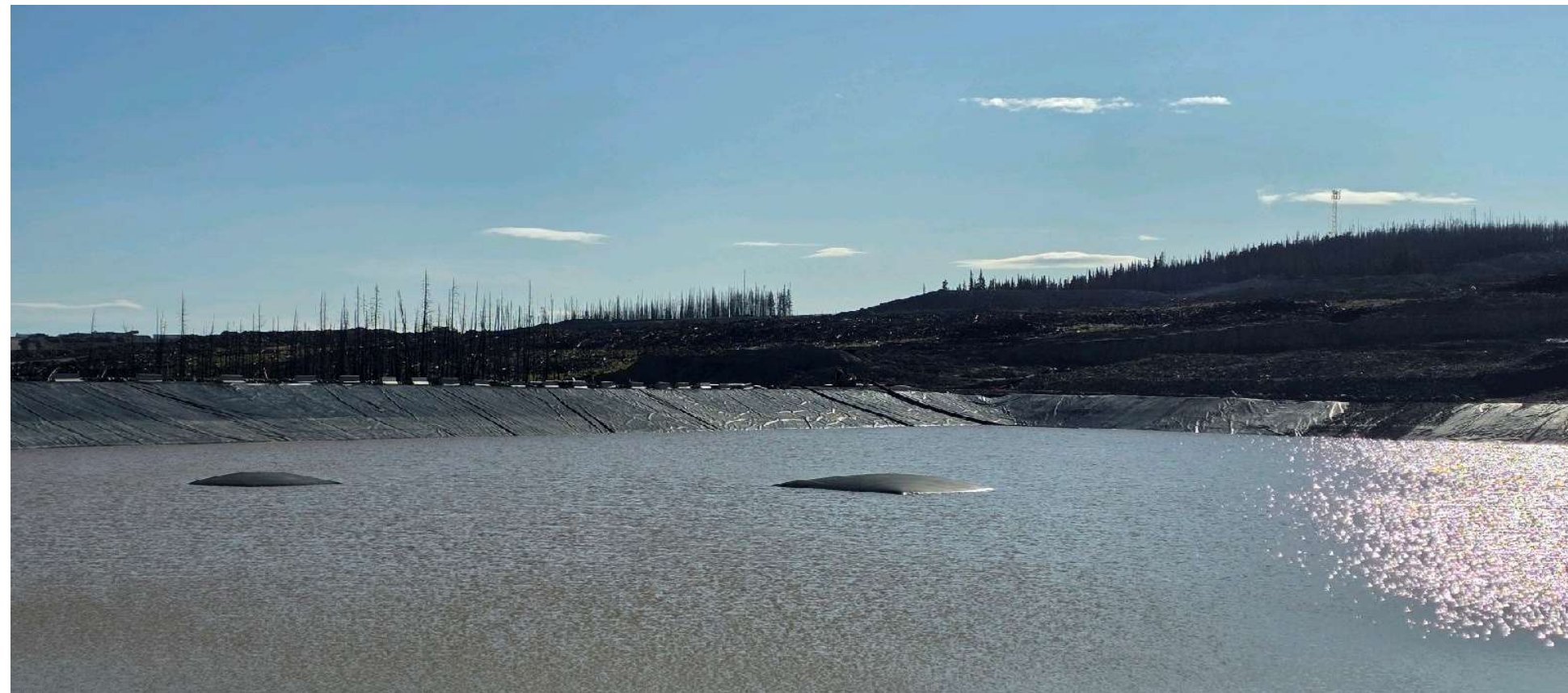
Photo 114220-1. Portions of the liner along the base of the LGO stockpile pond protruding in 'bubble-like' formations. BWG detailed the cause of the protrusions is trapped air beneath the liner and that there are no concerns with the integrity of the liner as confirmed by the Engineering departments.
