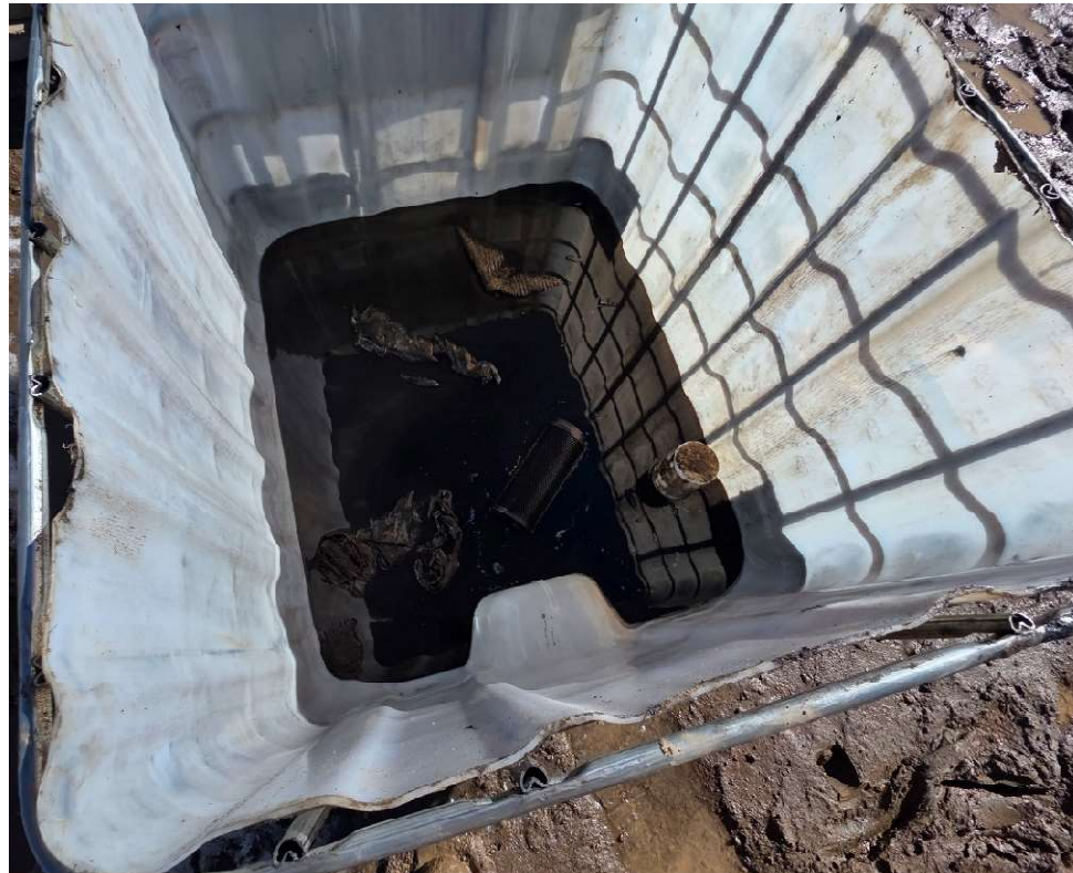
Photo 113521-5. Example of former storage tote being utilized as a drip tray containing used oil and oil filters at the mobile maintenance yard.
