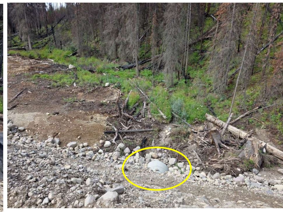
Photo 114199-1. Upstream side of culvert crossing of Watercourse 636 at 9.5km on the C-Trail access road.
