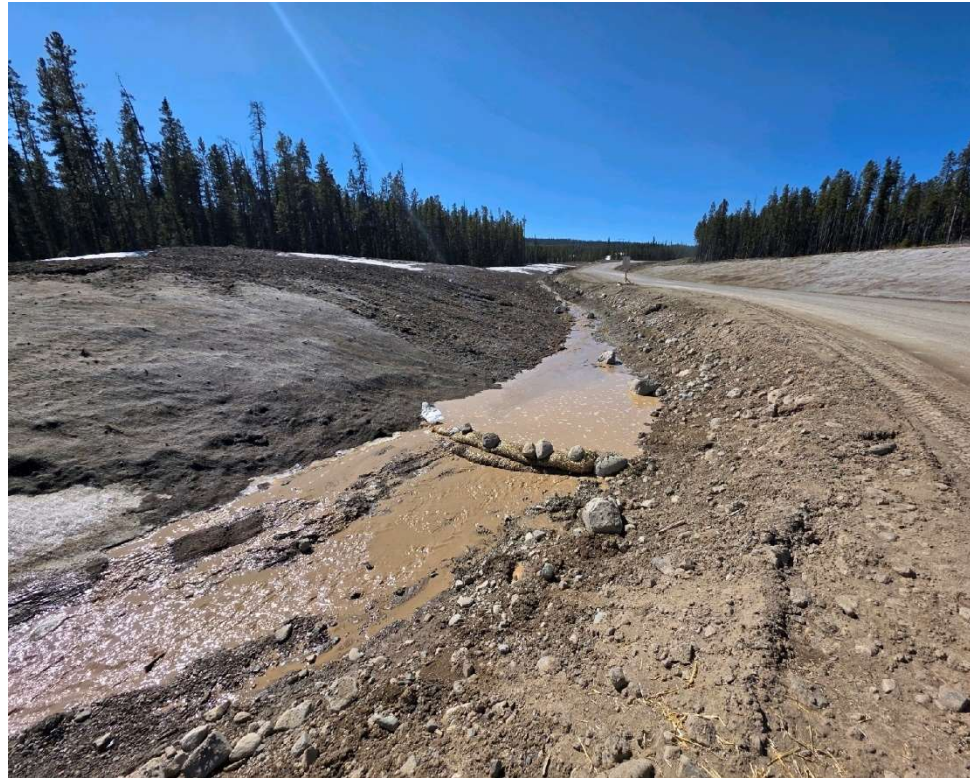
Photo 113513-9. Turbid water flowing in ditch line along road to Operations Camp. Water from ditch flowing into Watercourse 146 located downstream of this image (see photo 113513-10). Photo taken morning of April 15, 2025.
