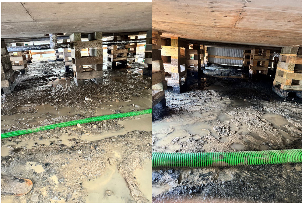
Photos 1 & 2: Spill Photos
