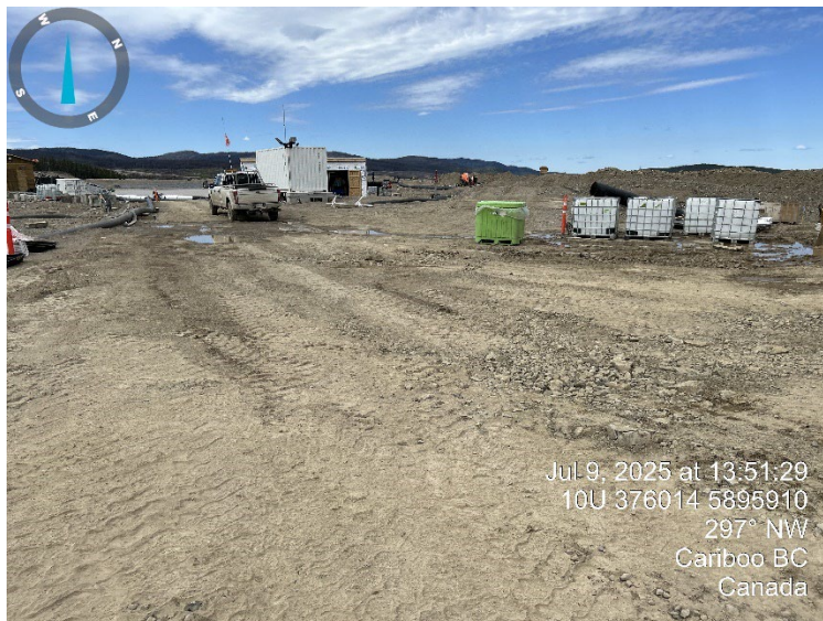
Photo 6: Spill Clean Up
