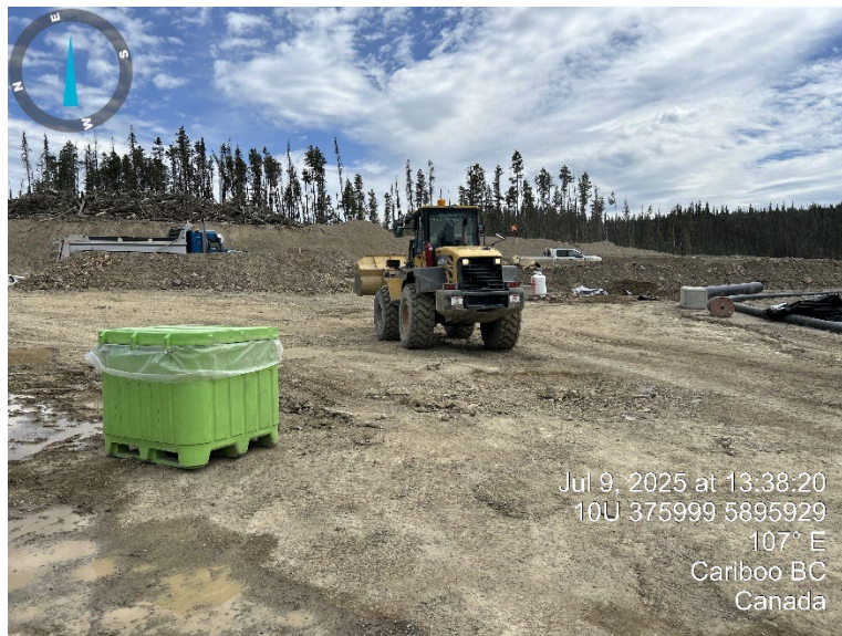
Photo 4: Spill Cleanup Ongoing
