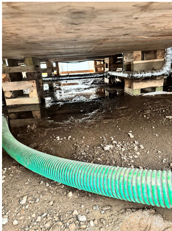
Photo 5: Spill Clean Up
