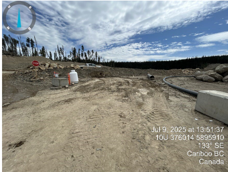
Photo 7: Spill Clean Up
