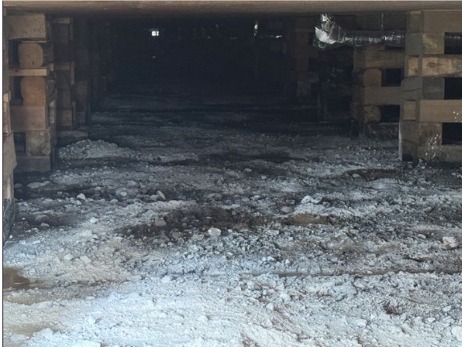
Photo 6: Spill Clean Up
